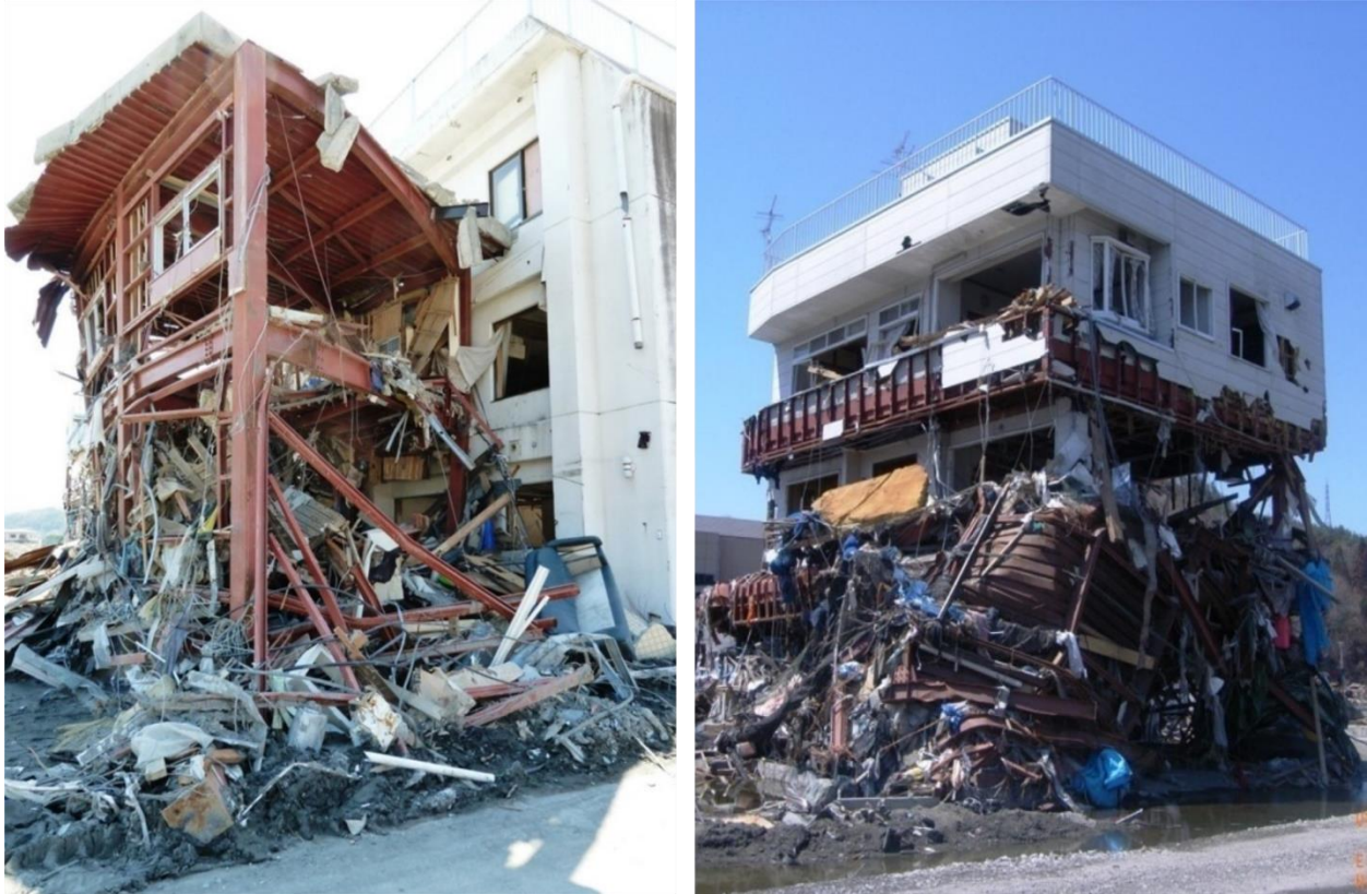
Figure 1.3: Photos of debris dams that had formed on structures after the 2011 Tohoku Tsunami (courtesy of Dr. Ioan Nistor).
