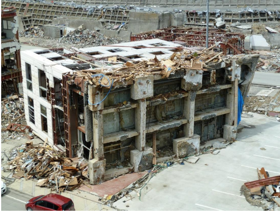
Figure 1.1: An overturned reinforced concrete structure in Onagawa, Japan, after the 2011 Tohoku Tsunami (courtesy of Dr. Ioan Nistor).
