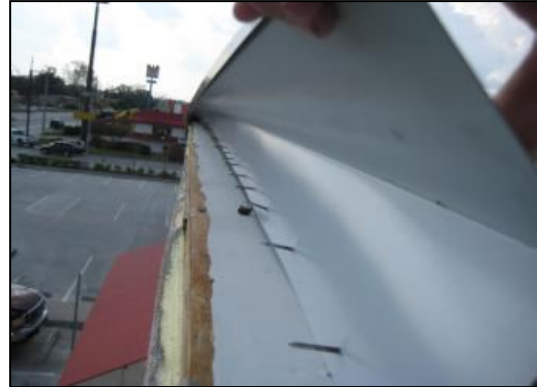
(b) Failure of edge flashing
