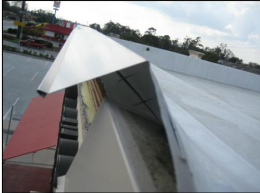
(a) Un-cleated edge flashing peeled off the edge
