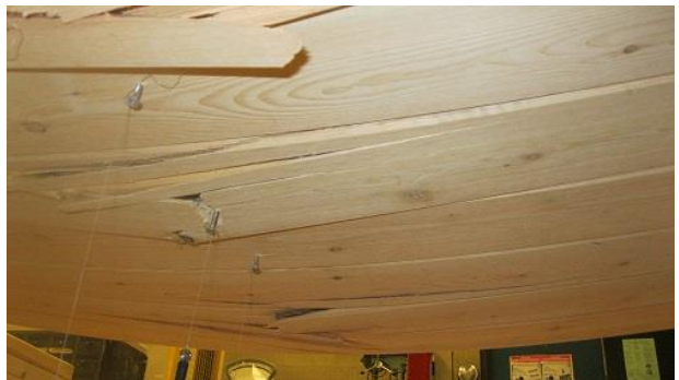
Simple Span 7 Board Failure
