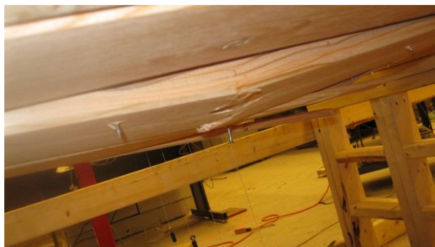
(a) Bending Failure
