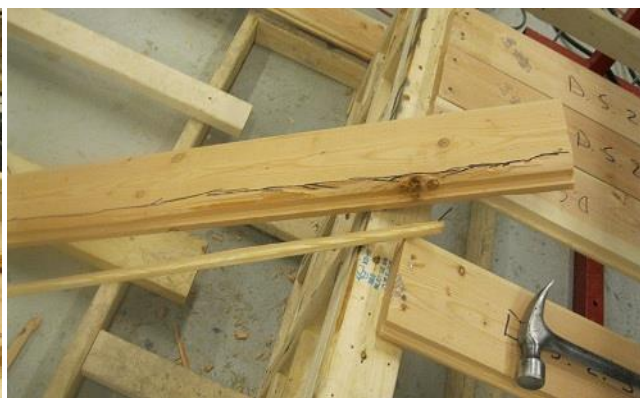
(b) 5 Board Failure (CL127)
