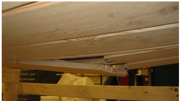
Simple Span 5 Board Failure
