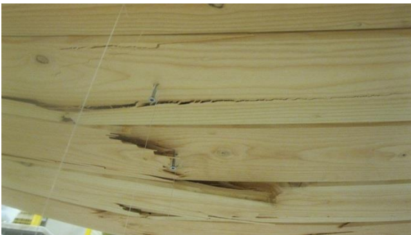
Simple Span 5 Board Failure
