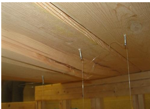
Simple Span 7 Board Failure with sheathing (Bottom View)
