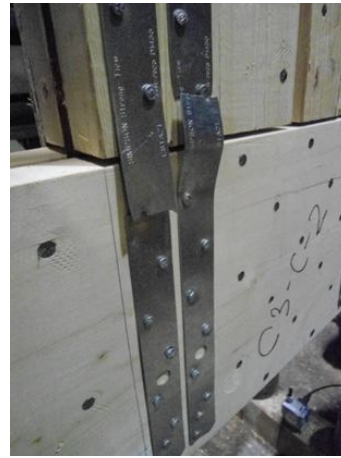
(b) Metal strap failure right face
