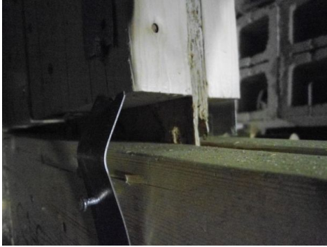
(a) Middle OSB failure and Metal strap failure left face
