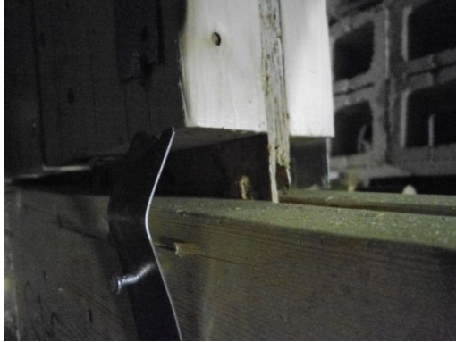
(a) Middle OSB failure
