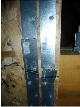
(a) OSB and metal strap failure left face
