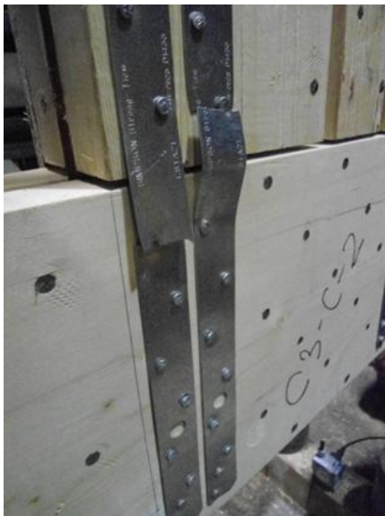
(c) Metal strap failure
