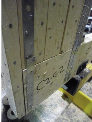
(a) Metal strap failure left face
