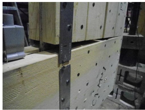
(b) Metal strap failure right face
