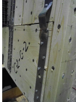
(b) Metal strap failure right face
