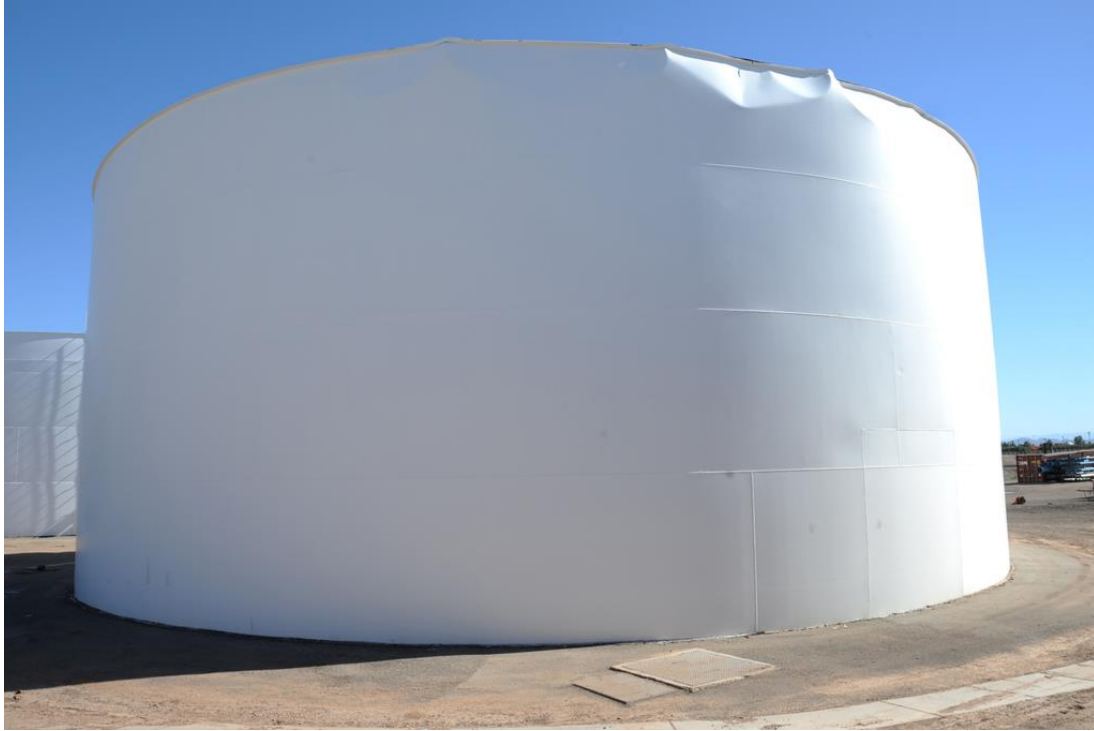
Figure 1- 4 Damages to liquid tanks during 2010 Calexico earthquake in California ( http://www.fema.gov/media-library/assets/images/56703 )
