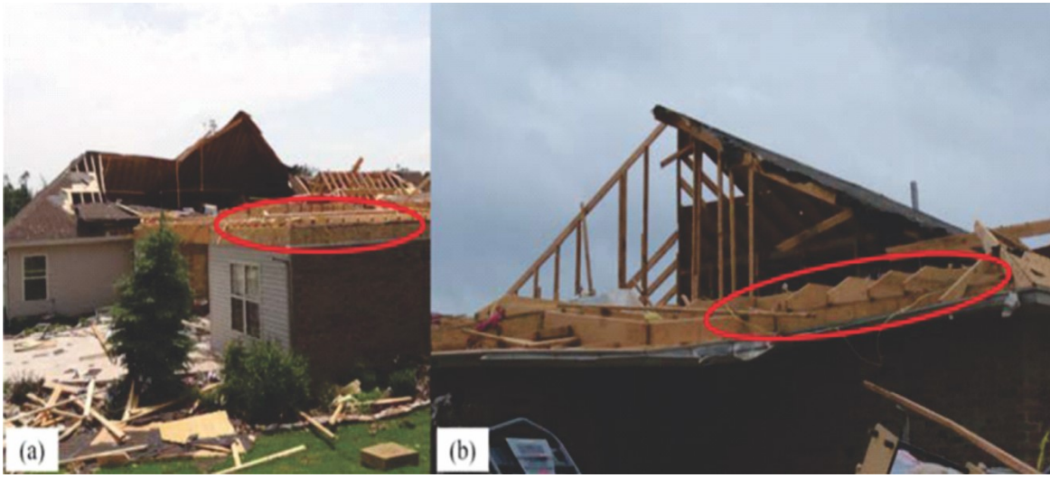
Figure 2. 21 Example of structural failures of roofs where the roof assembly was blown away [20]
