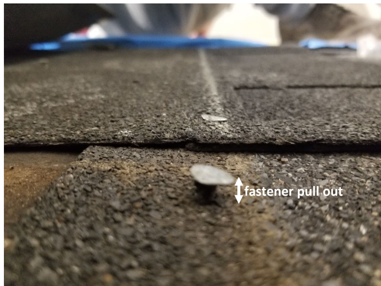
Figure 5.21 Fastener pulled out from deck and shingle tearing around fastener (Failure Mode2)
