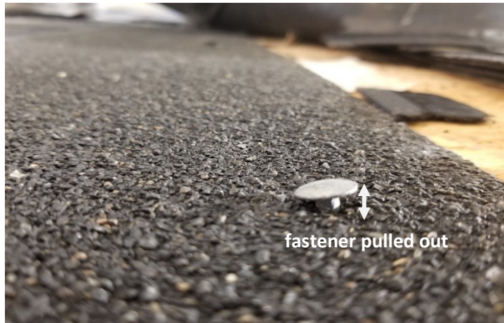
Figure 5.19 Fastener lifted from the shingle (Failure Mode 2) of the field zone mock-up
