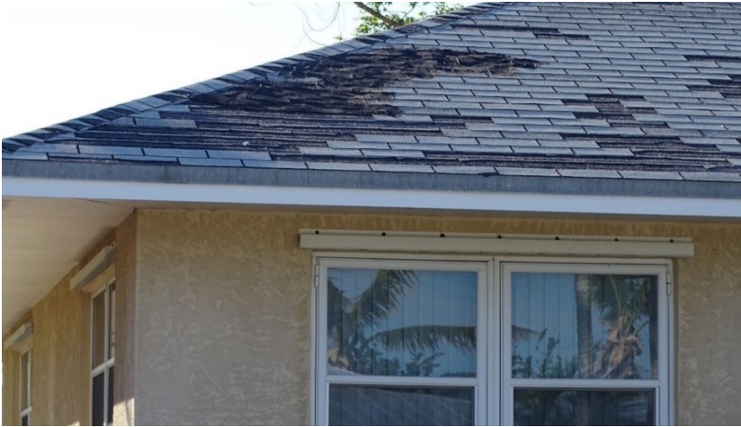
Figure 2. 23 Example of shingles blow off after a wind event in Ottawa 2020, [36]
