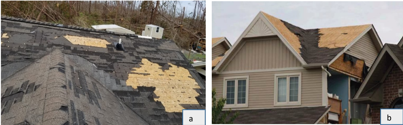
Figure 2. 24 Shingle blow off with peeled underlayment after a wind event in Ottawa 2020 [36] (a) and Angus [4] (b)
