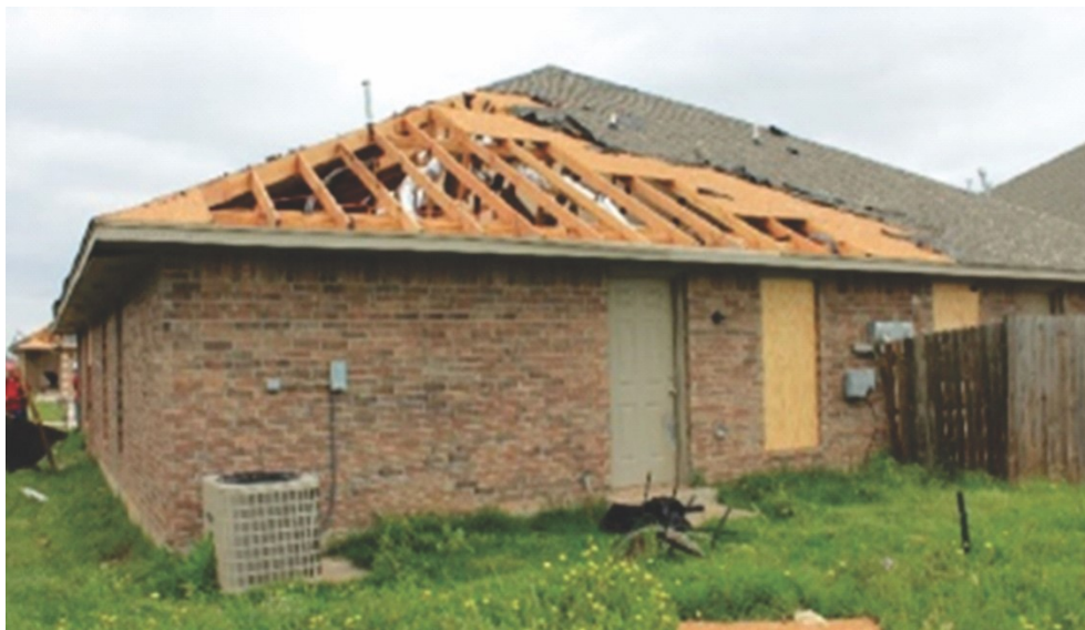
Figure 2. 22 Example of structural failure of the roof where the deck sheathing was blown away [35]
