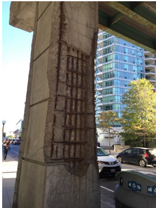
Figure 2.15: Cover delamination on pier of Gardiner Expressway - Toronto, ON
