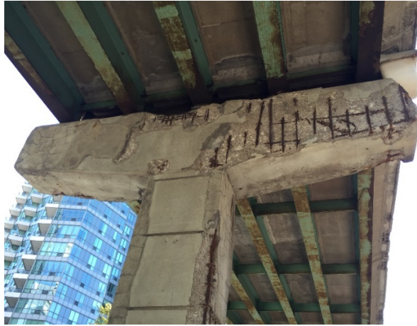
Figure 2.14: Cover delamination on cap beam of Gardiner Expressway - Toronto, ON
