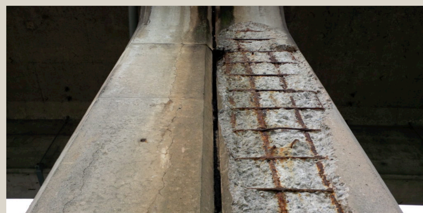
Fig. 1: Corroded reinforced concrete member
