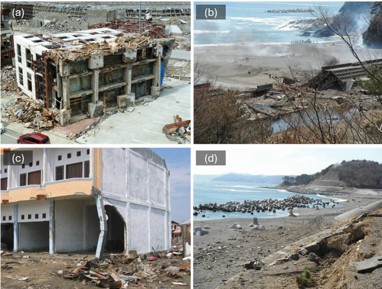
Figure 7: various examples of infrastructure failure that occurred during past tsunami events; (a) Overturned reinforced concrete/steel building in Onawaga, March 2011; (b) breached coastal protection dyke near Hachinohe, Japan, March 2011; (c) debris impact on a column, Banda Aceh, December 2004; (d) damaged coastal protection revetment, near Hachinohe, Japan, March 2011 (courtesy of Ioan Nistor)
