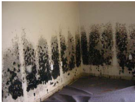
Figure 2.12. Fungal growth on indoor drywall material [22].
