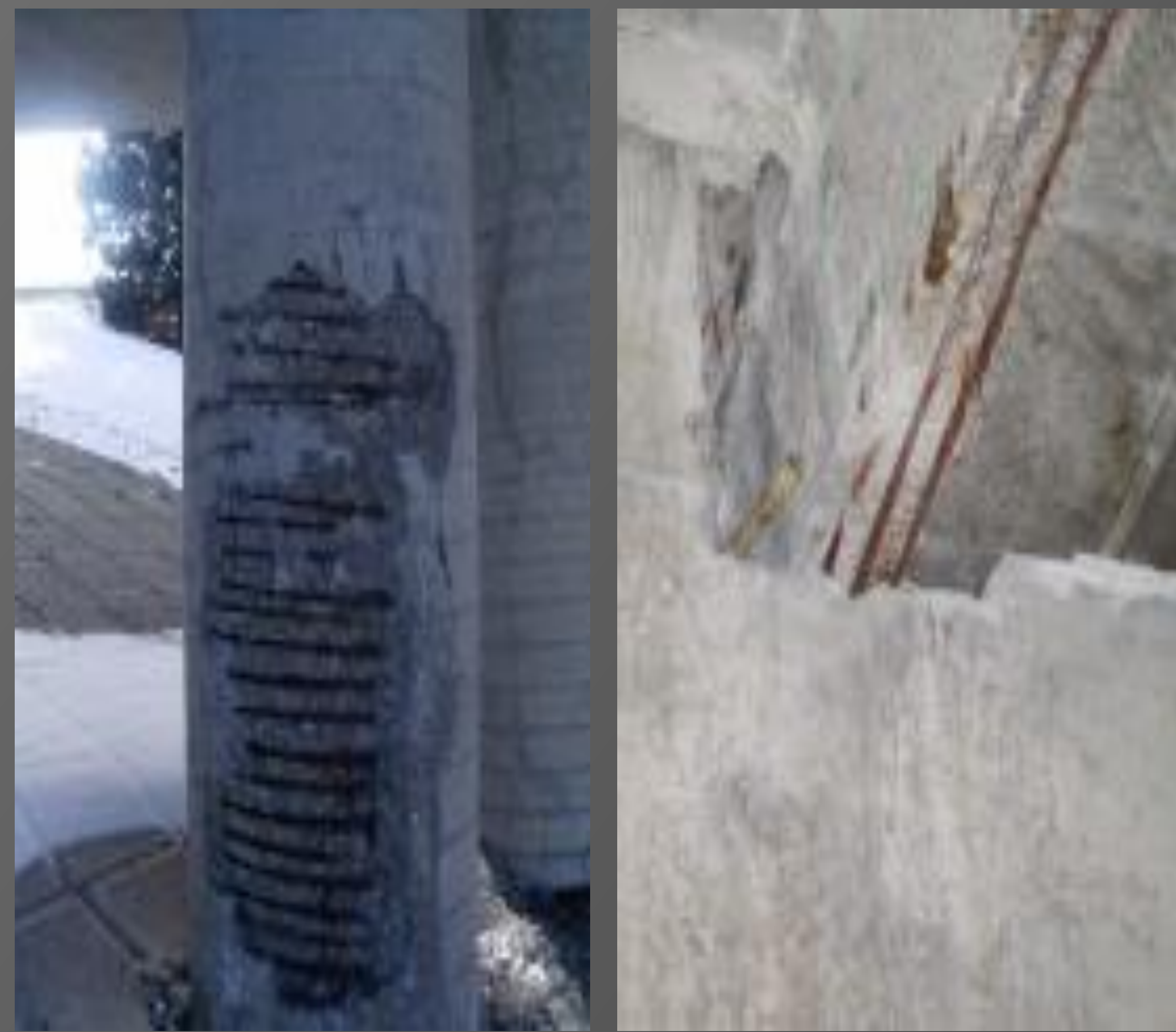
Fig 1: Reinforced concrete elements affected by corrosion
