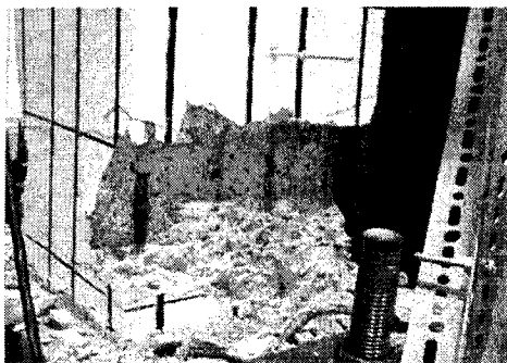
(f) Column Failure
