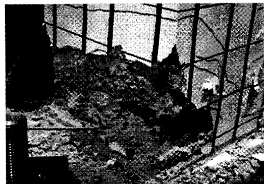
(f) Column Failure
