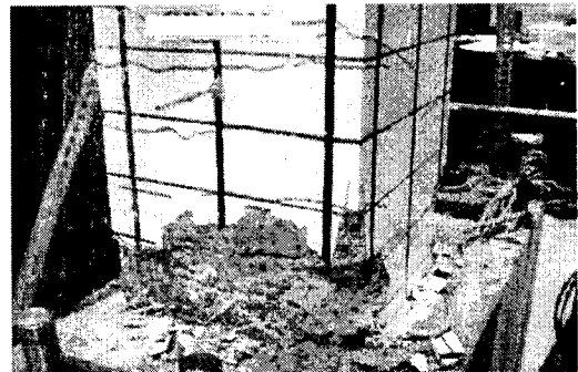
(f) Column Failure
