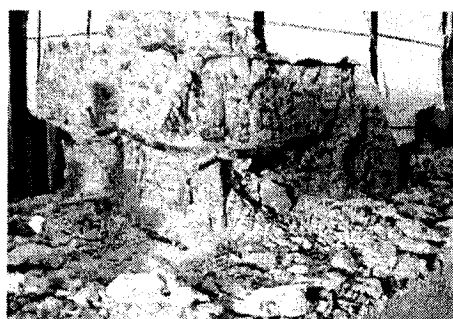
(f) Column Failure
