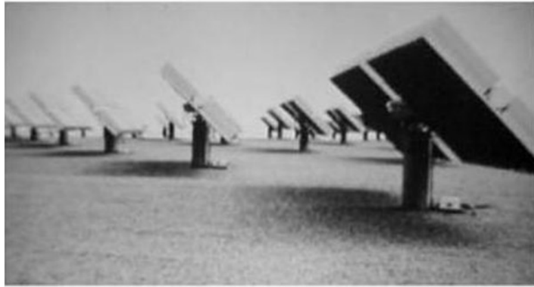
Figure 3 The 350kWp SOLERAS project in Saudi Arabia [4].
