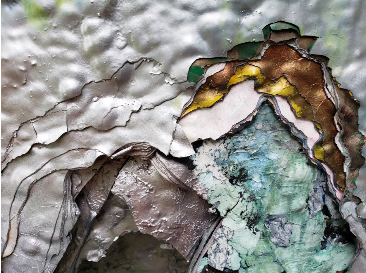
Figure 23. Peeling Layers of Paint (Campbell, photograph, 2018)
