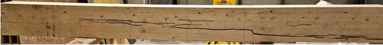
a) Cracks along the glulam layers
