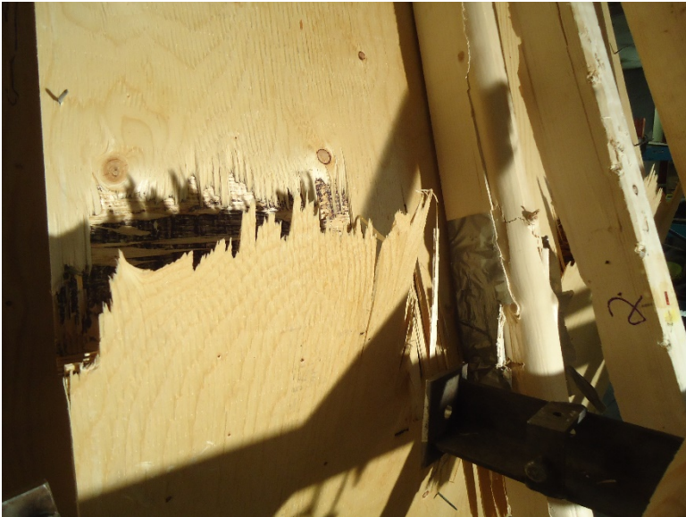
c) Damage to plywood panel
