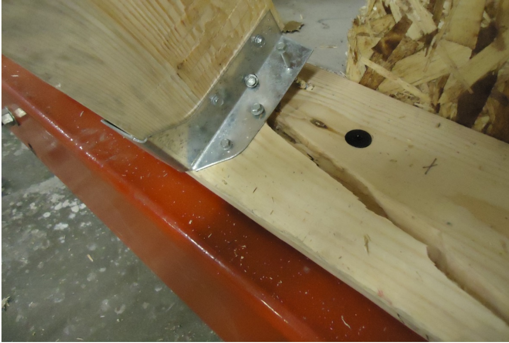
Figure 6.16 : Typical connection damage for HU28 connections
