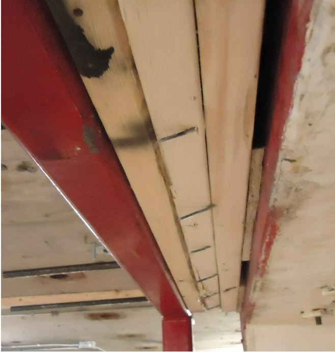
A. Nail-withdrawal failure at top blocking
