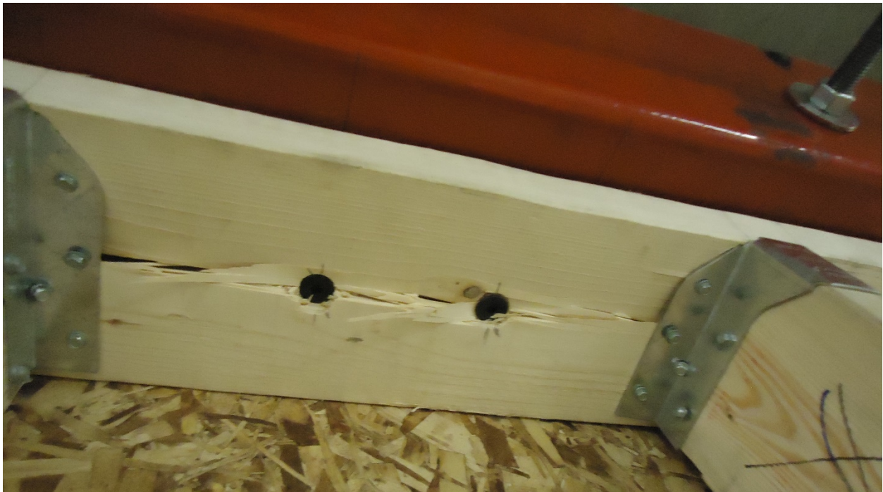
Figure 6.19 : Damage in top plate in wall with LJS26DS
