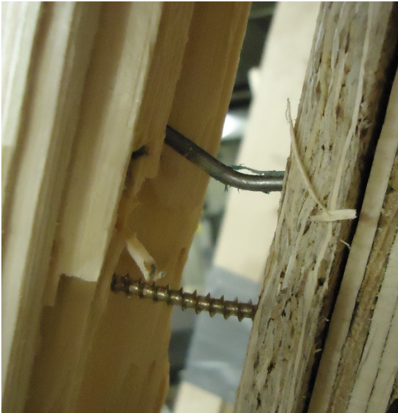
b) Exposed fasteners at Stud 1
