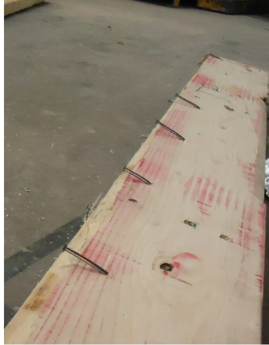
B. Nail puncture failure at top plate
