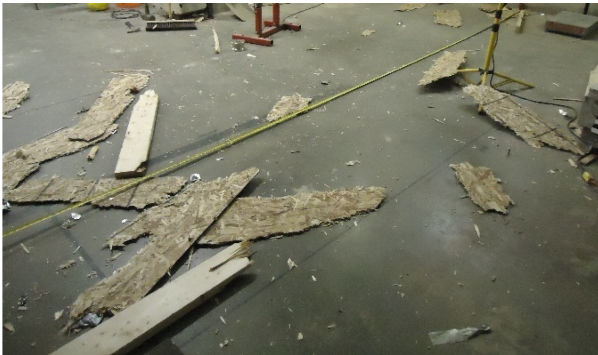
c) Wall debris
