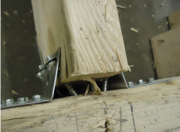
A. LJS26DS connection damage
