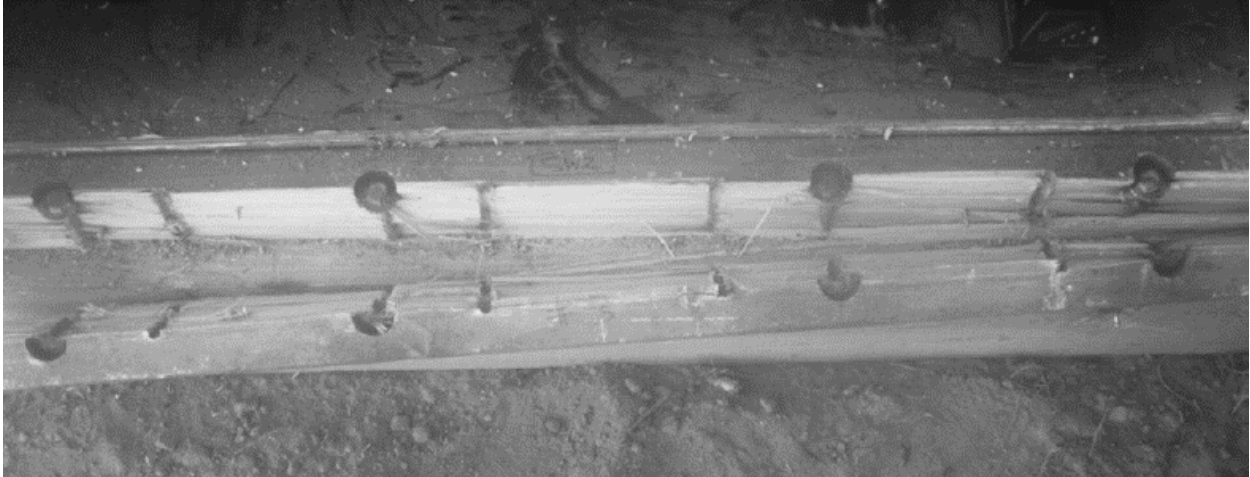
Figure 2.1 : Damaged CSL connection plates (Syron, 2010)
