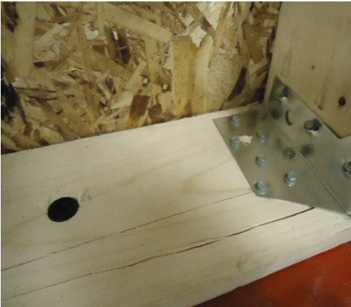
c) Damage to bottom plate
