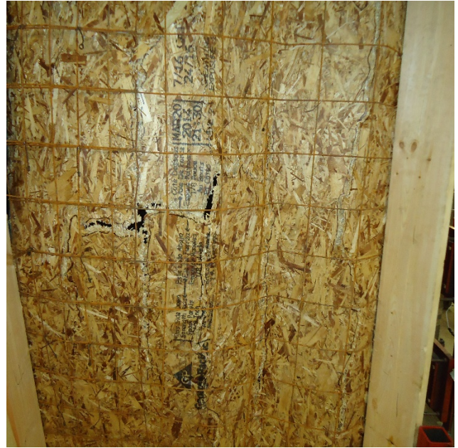
b) Damage to OSB and WWM
