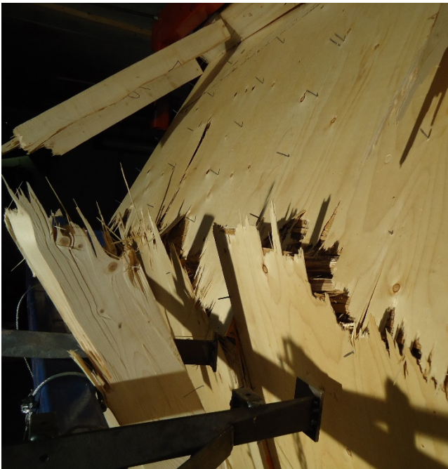
b) Damage to sheathing and exposed nails
