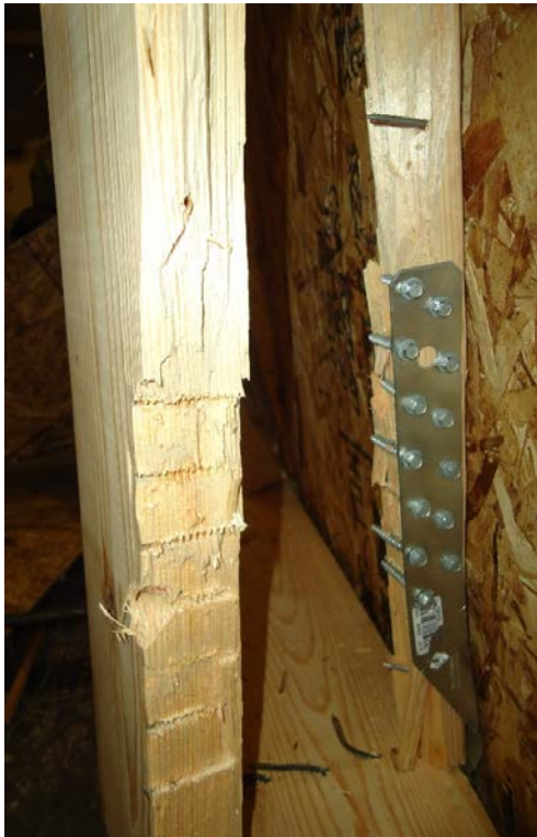
A. Splitting failure
