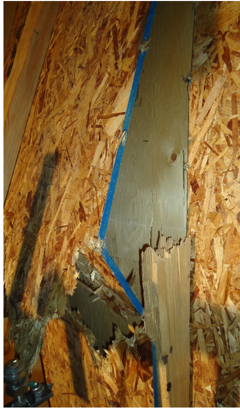
c) Damage to OSB panel
