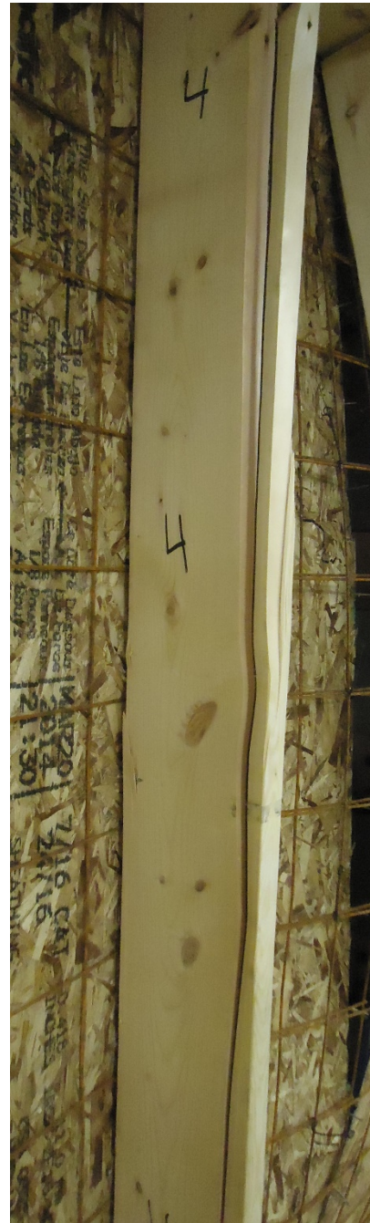
c) Superficial damage to Stud 4
