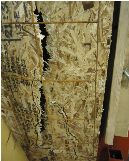
b) Damage to OSB
