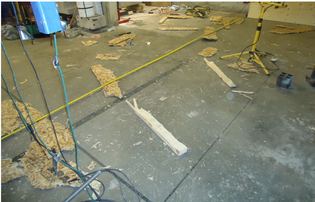
c) Wall debris
