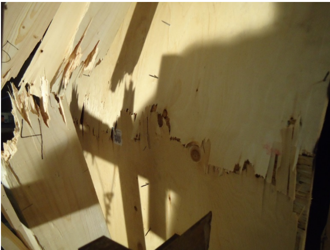
b) Damage to sheathing and exposed nails
