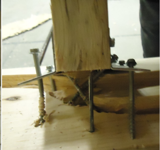
B. HU28 connection damage
