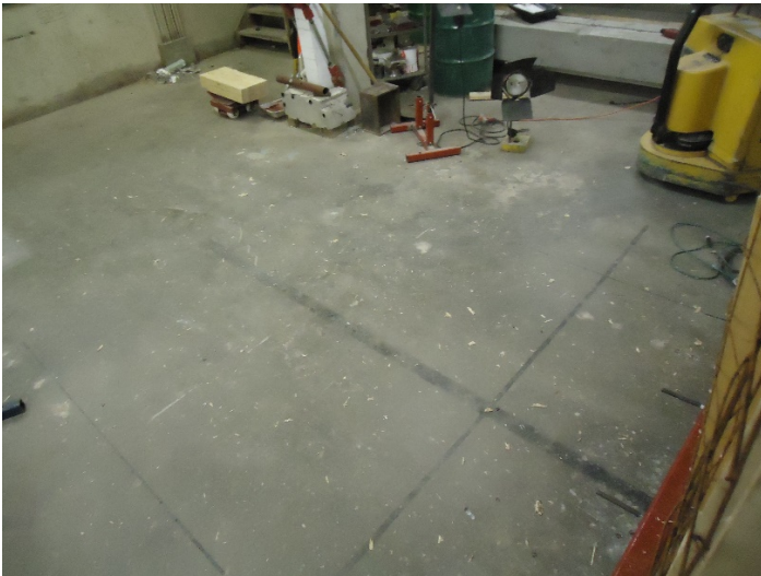
b) Lack of noticeable debris
