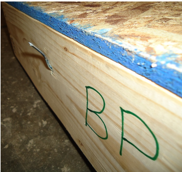
c) Nail yielding and withdrawal at bottom plate
