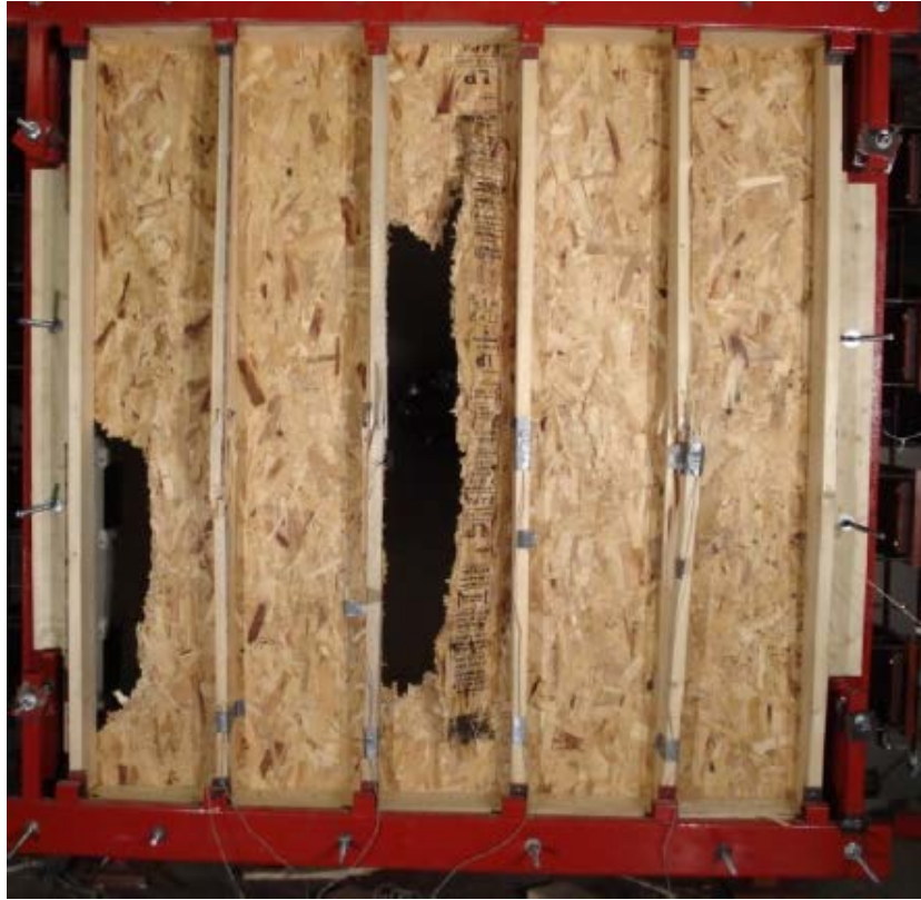
Figure 2.3 : Damaged OSB sheathing (Lacroix, 2013)
