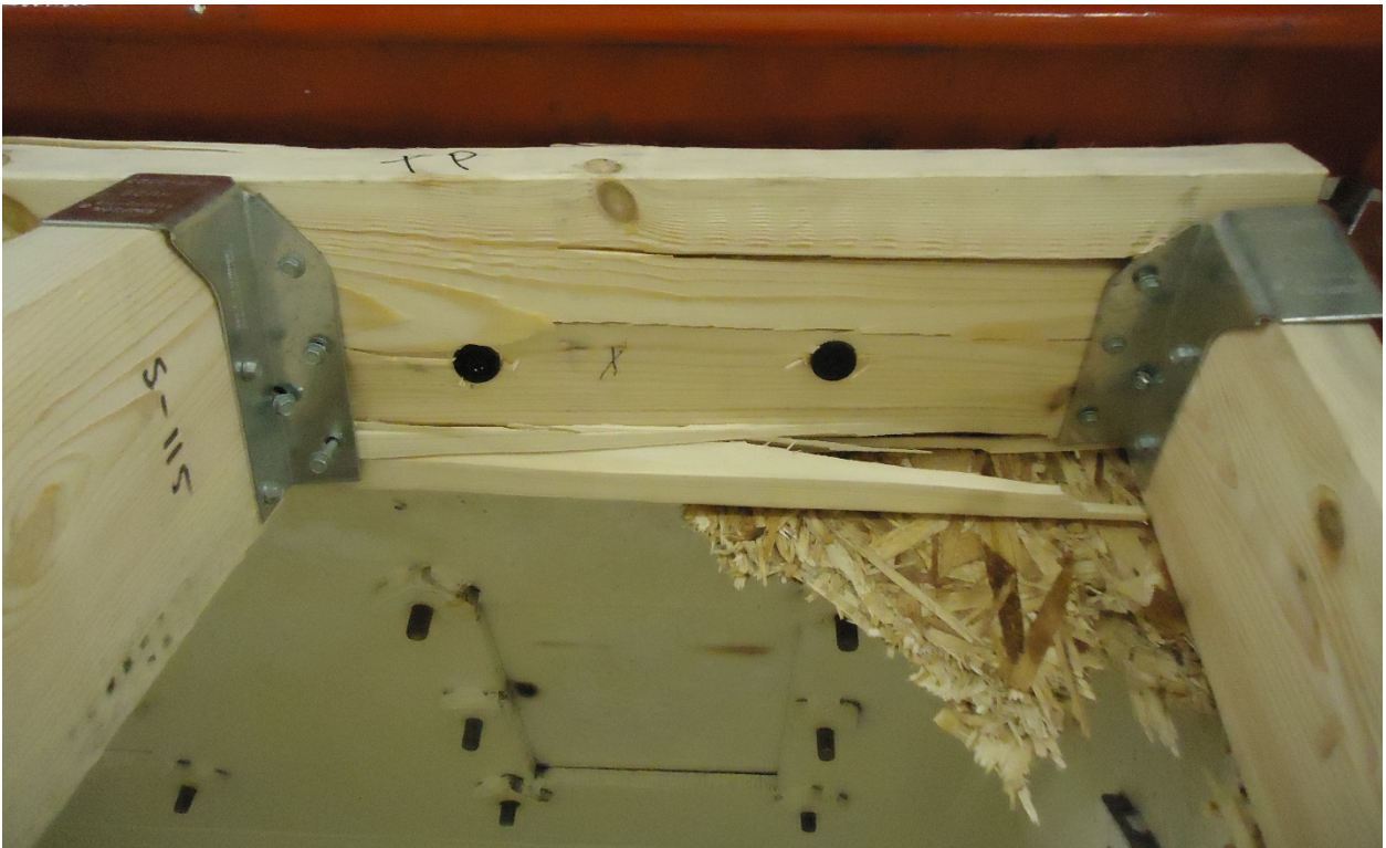
c) Damage to top plate between Stud 1 and 2
