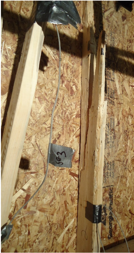
b) Failure of stud 2 caused by fastener tips
