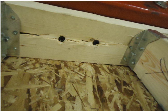
c) Damage to top plate
