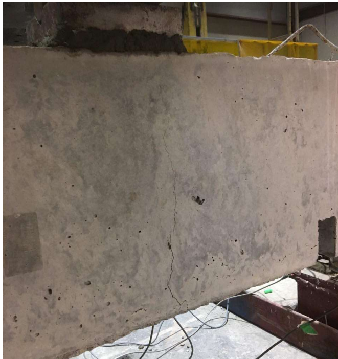
Figure 4.9 First Flexural Crack
