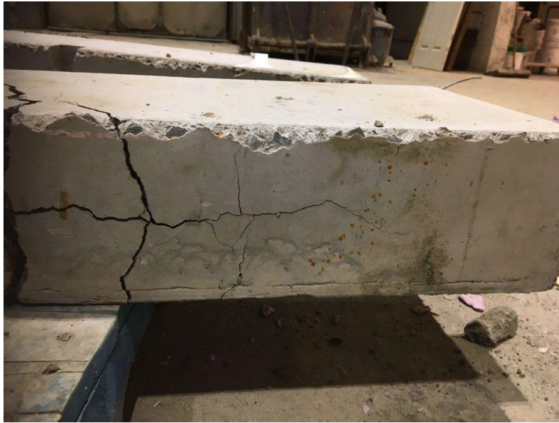
Figure 4.10 Longitudinal Crack Propagation
