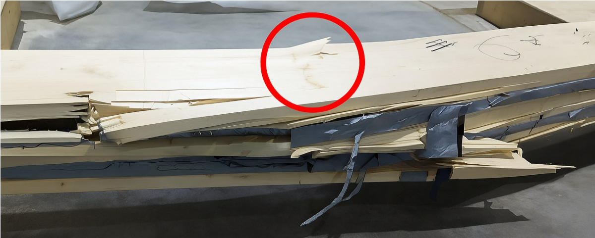
b) Damaged reinforced beam
