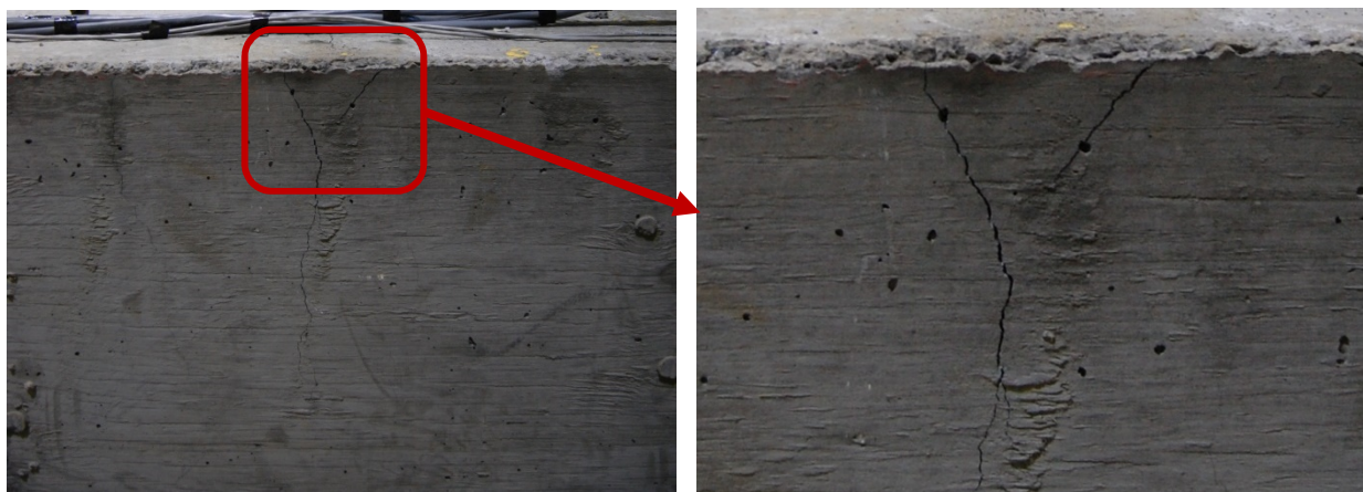
Figure 5.30 Shear Wall No. 2 – Visual Signs of Foundation Cracking
