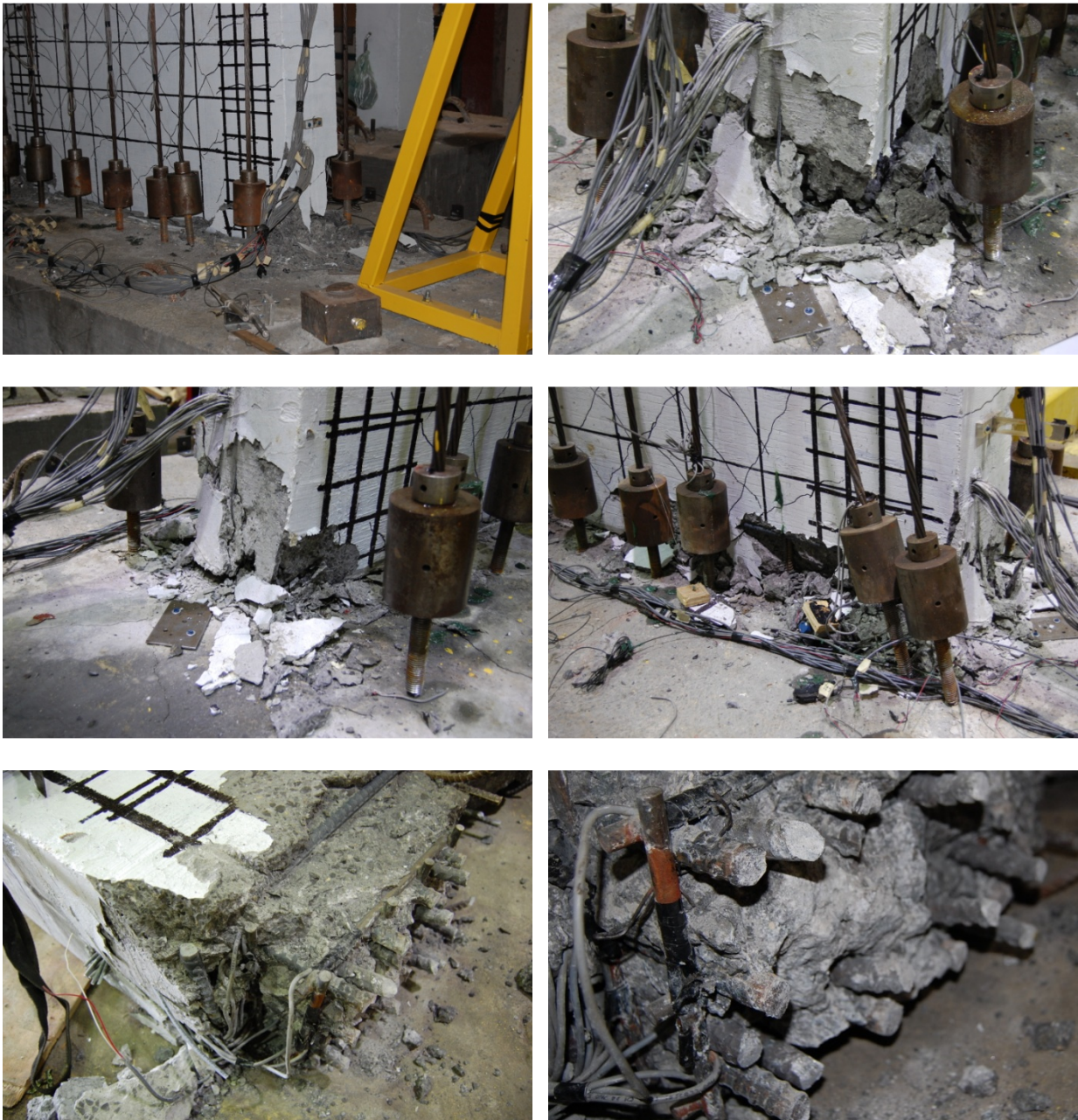
Figure 5.25 Shear Wall No. 2 Failure Photos (bottom two after the failure, when the wall was turned over to expose the bottom section)
