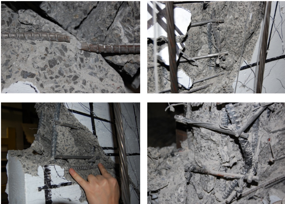
Figure 5.12 Shear Wall No. 1 Failure Photos
