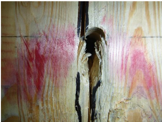
(c) Crushing at bolt hole edge
