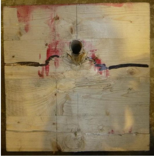
(a) No splitting failure
