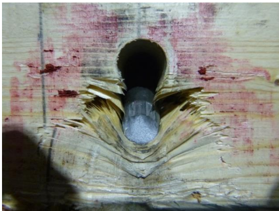
(c) Crushing at bolt hole edge
