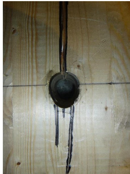
(b) Crushing in bolt hole
