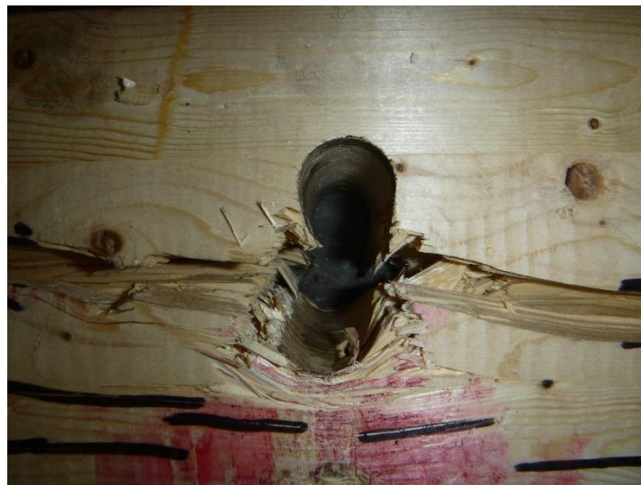
(b) Crushing in bolt hole
