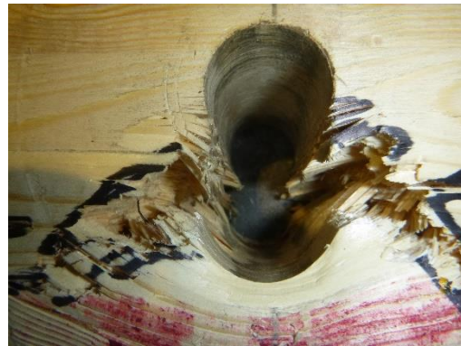
(b) Crushing in bolt hole
