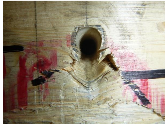
(b) Crushing at bolt hole edge
