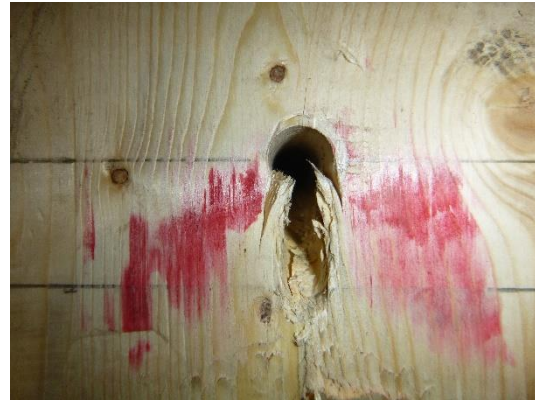
(b) Crushing at bolt hole edge
