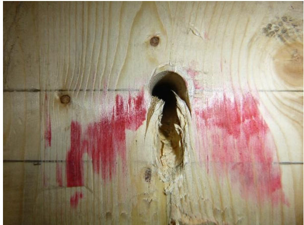
(b) Deformation in bolt hole
