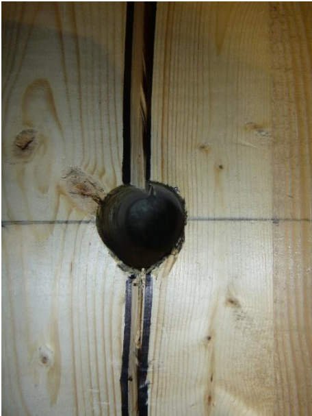
(b) Crushing in bolt hole
