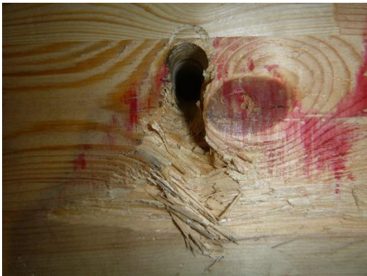
(c) Crushing at bolt hole edge
