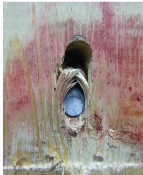
(b) Crushing at bolt hole edge
