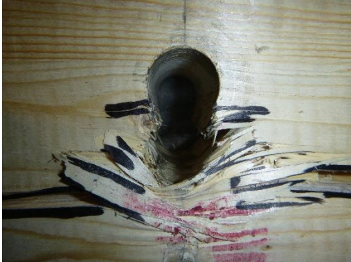
(b) Crushing in bolt hole
