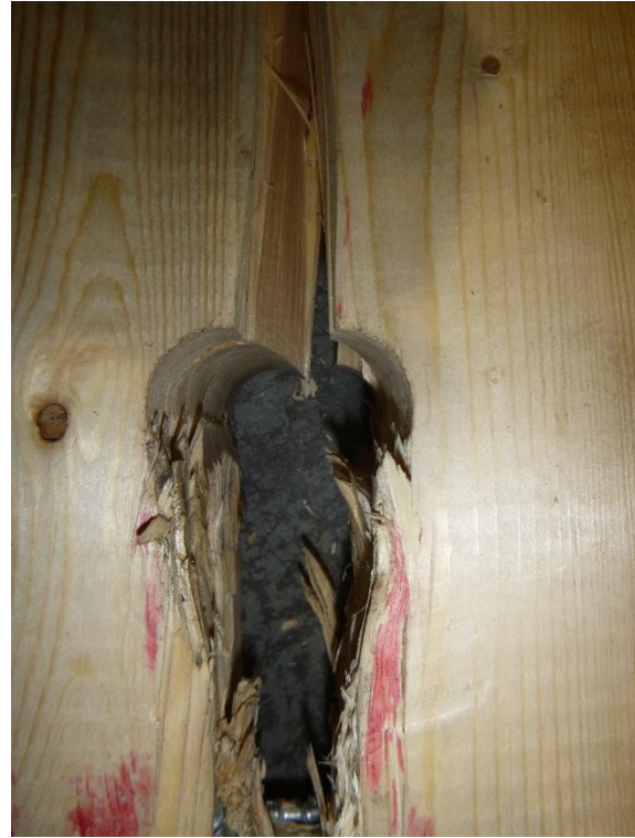
(b) Extensive crushing in bolt hole before splitting
