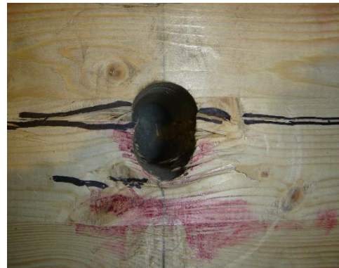
(b) Crushing in bolt hole
