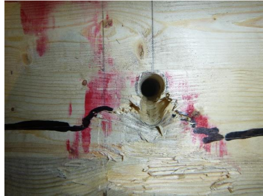
(b) Crushing at bolt hole edge
