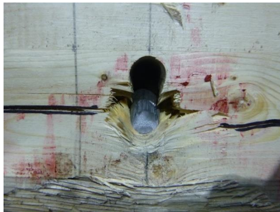
(c) Crushing at bolt hole edge
