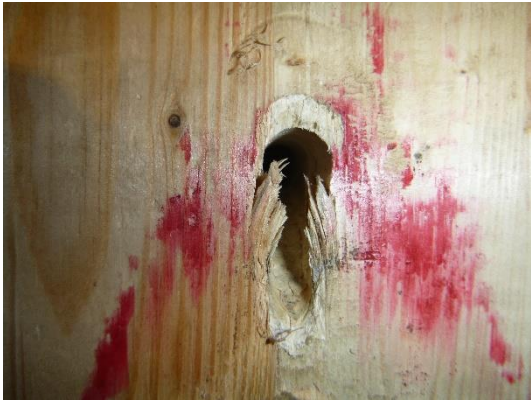
(c) Crushing at bolt hole edge
