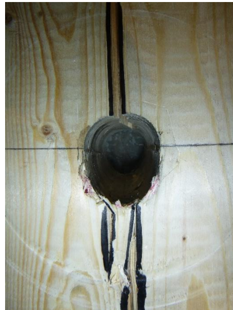
(b) Crushing in bolt hole
