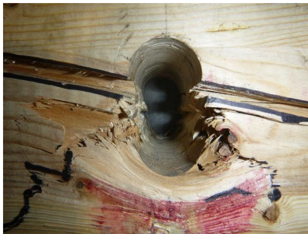
(b) Crushing in bolt hole
