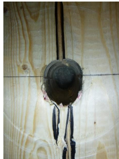
(b) Crushing in bolt hole
