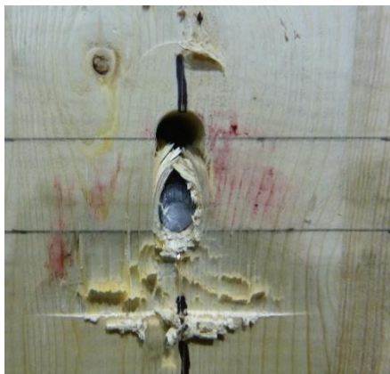
(c) Crushing at bolt hole edge
