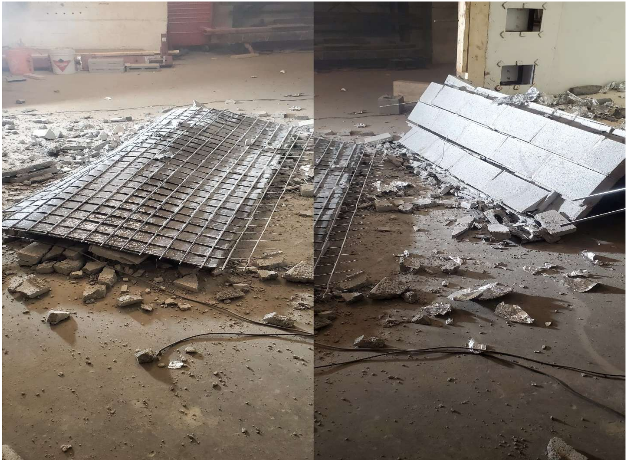
Figure 4.38. The collapse of Wall-3-5 with the release of debris
