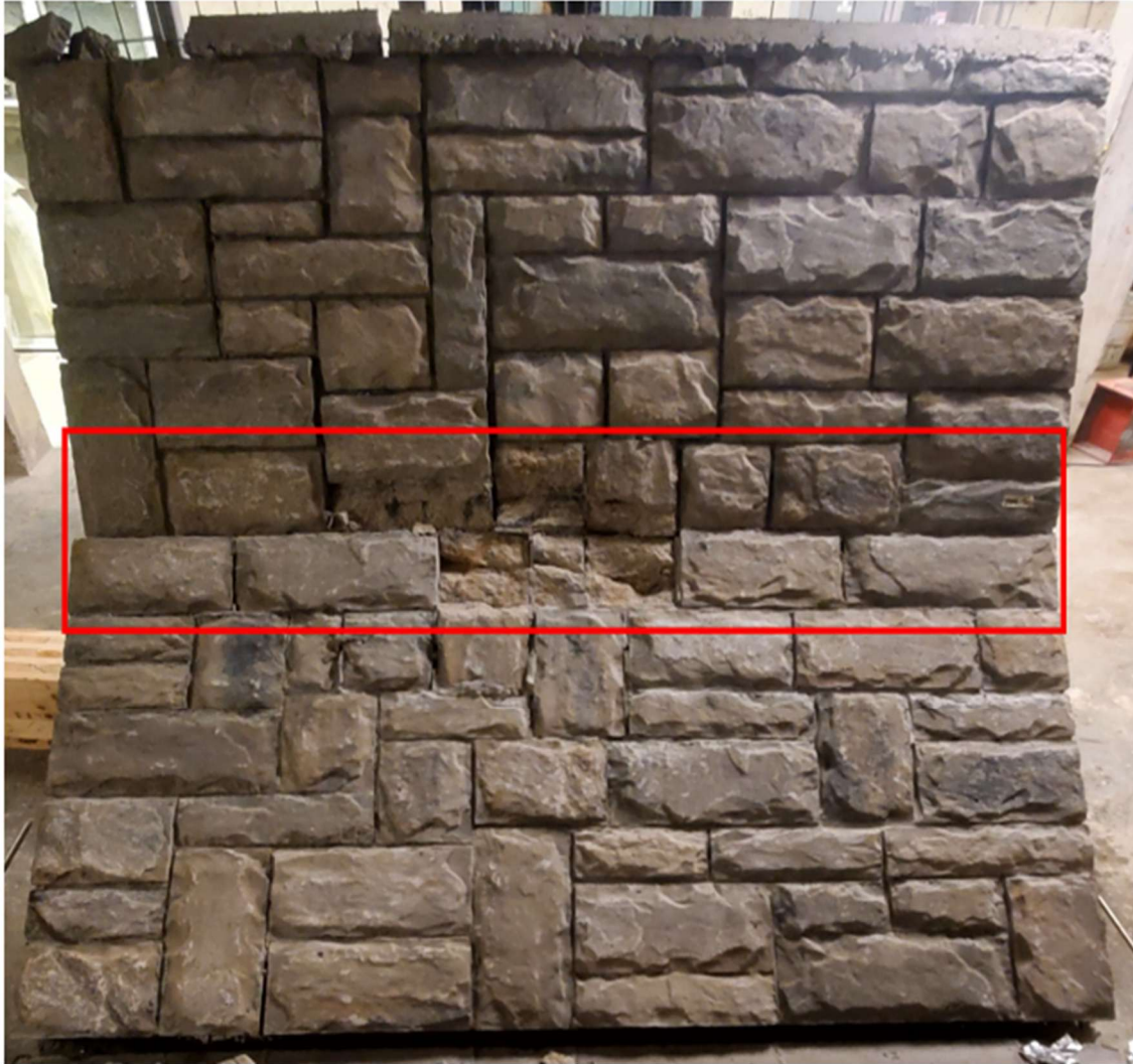
Figure 4.51. The exterior face of the failed Wall-4-5
