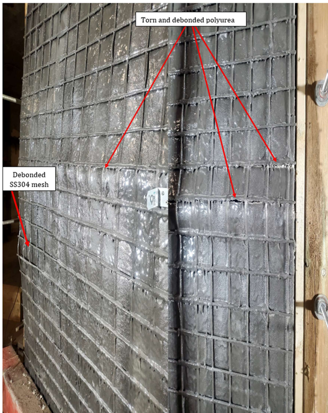
Figure 4.35. Torn and Partially debonded reinforced polyurea retrofit on Wall-3-4
