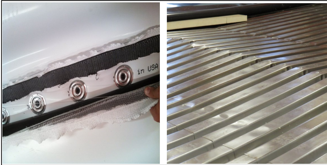
Figure 1.2 Roofing system failures: a) Failure in membrane. b) Deck buckling under wind pressure at fasteners row attachment
