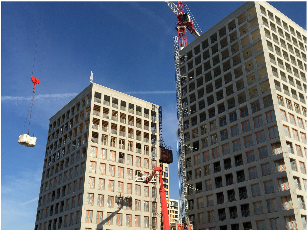
[Figure 13. Construction of the Chapelle International urban development near Porte de La Chapelle. This project is part of a large-scale rehabilitation of aging social housing and disused railway infrastructure from the Porte de Saint-Ouen to the Porte de La Villette. Photo by Author.]
