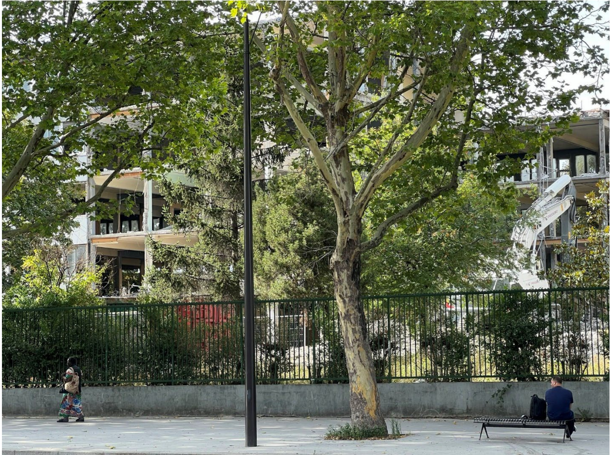
[Figure 5. Renovation of the Collège Maurice Utrillo on Boulevard Ney. Photo by Author.]
