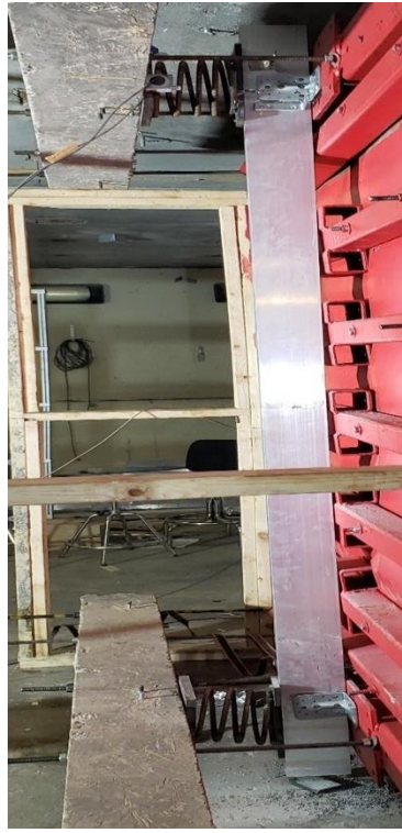
(b) Supports with spring dampers (MC-7)
