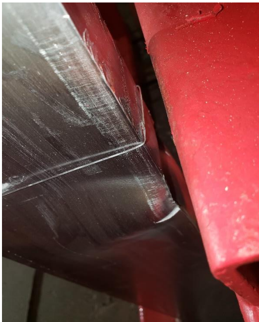
a) Local compression buckling
