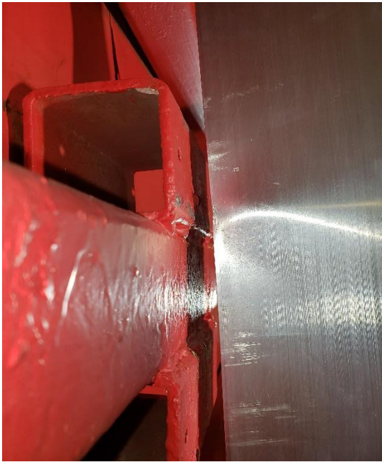
a) Compression buckling upper section
