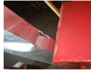
Flange buckling and failure
