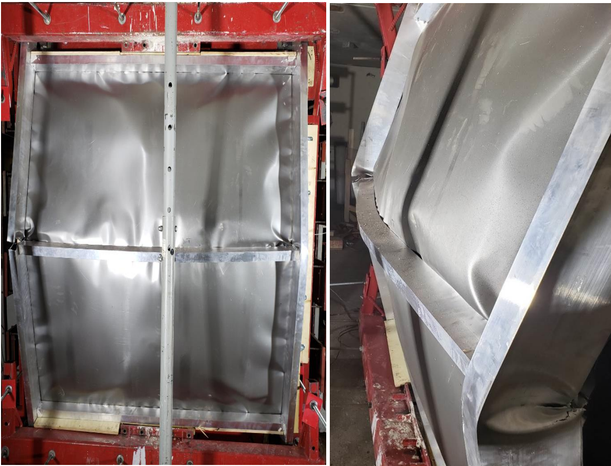
Figure 3.11: First curtain wall after blast test
