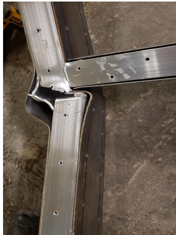
b) The core-aluminum failure
