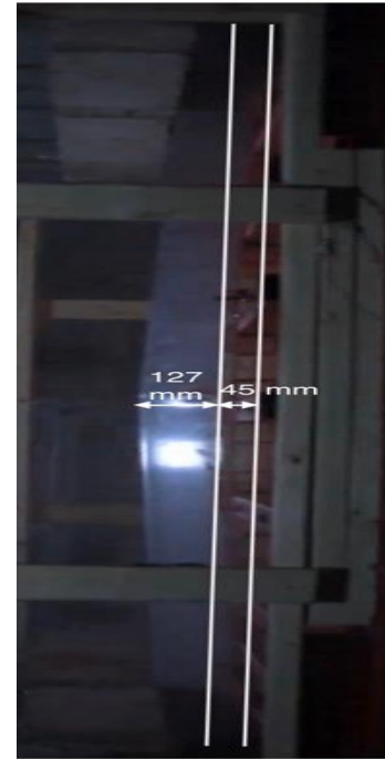
c) Residual deflection
