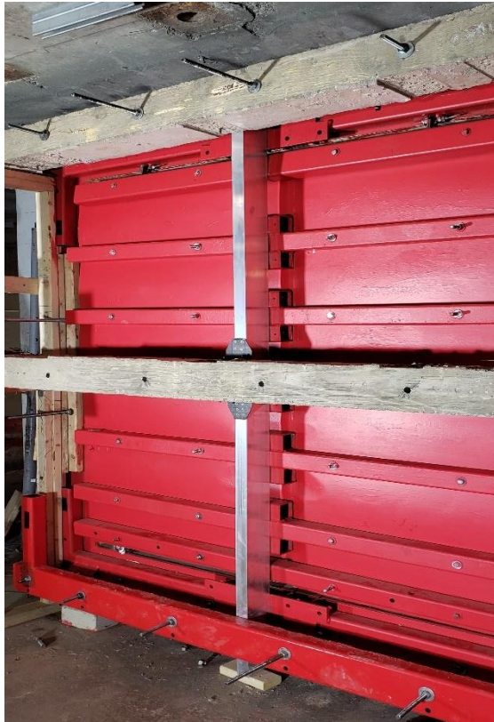
a) Overall view of test configuration
