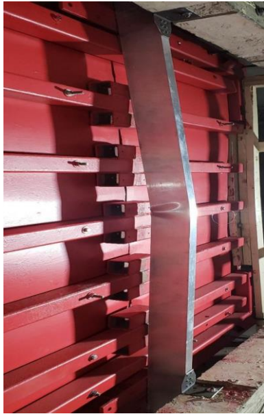
Bending of brackets at the ends
