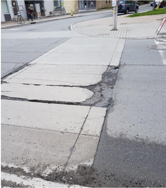
Figure 3: Crosswalk in participant’s neighbourhood – The participant explained that this crosswalk, right outside her building, had been in this state for a long time. Due her disability, it made it very difficult for her to cross the street in a timely manner for fear of falling.
