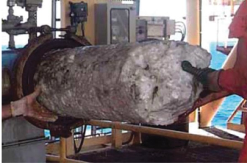
Figure 4-1. Pipeline blockage caused by gas hydrates. 9
