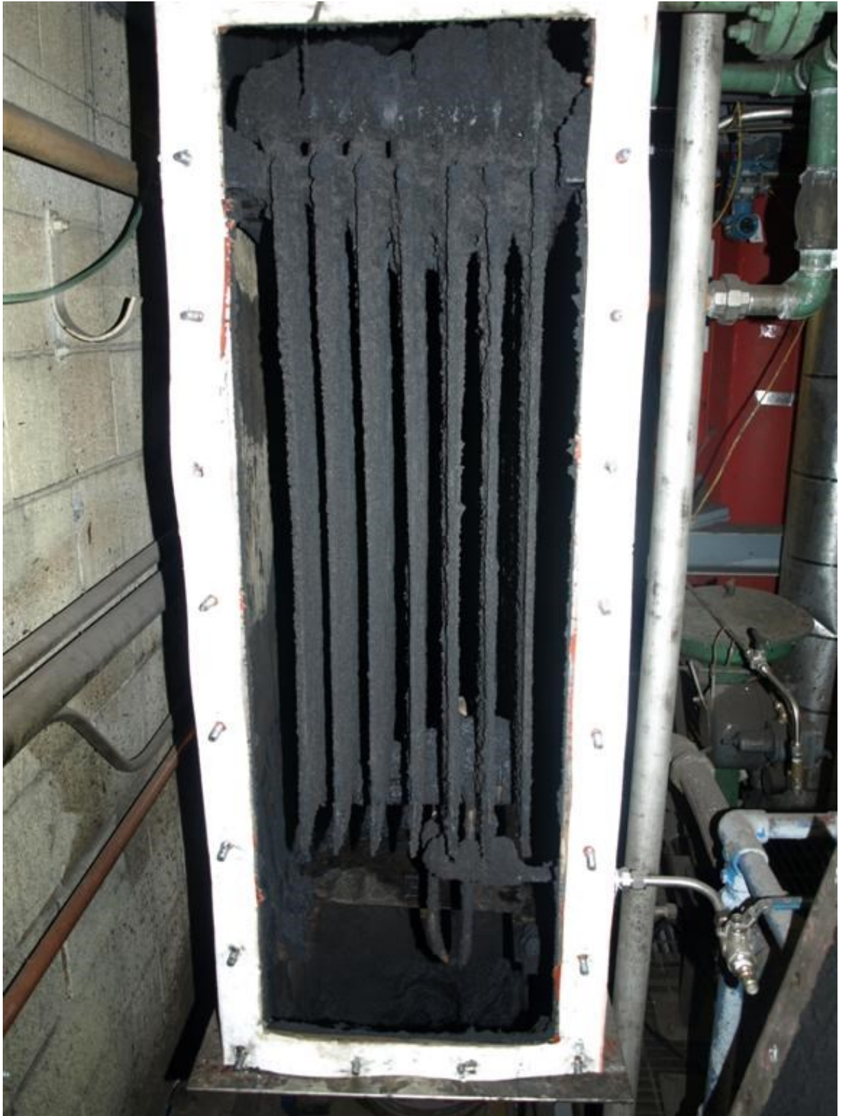
Figure E.6: Char / tar accumulation in the condenser from the large pilot-scale gasifier
