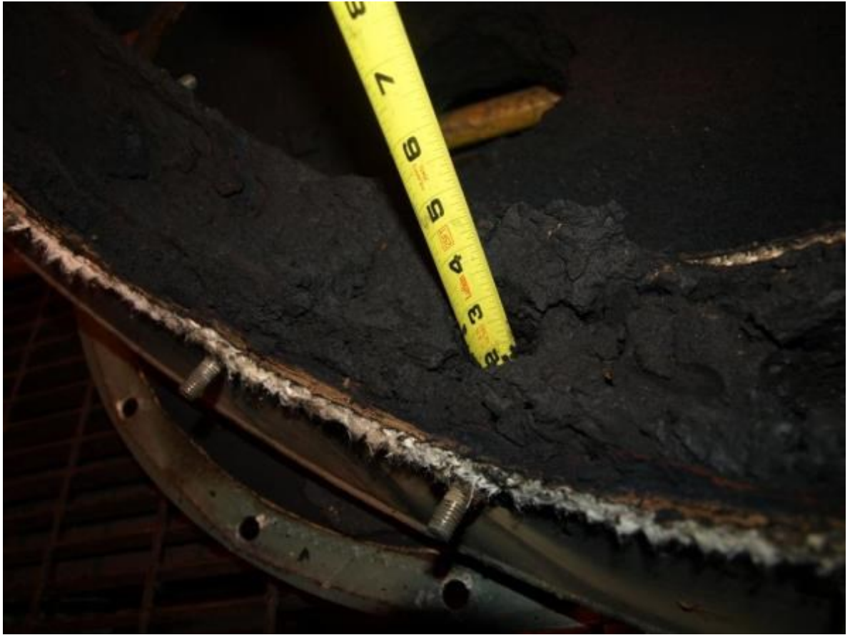
Figure E.7: Char / tar fouling found in the gas blower housing from the large pilot-scale gasifier
