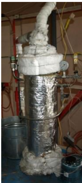
Figure E.2: "Tar Trap" from the gas sampling system installed in the small pilot-scale gasification facility
