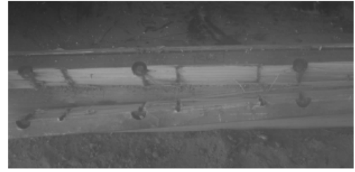
(b) Damage to connection plate
