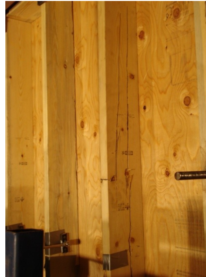
(b) Localized damage stud 5-Upper half
