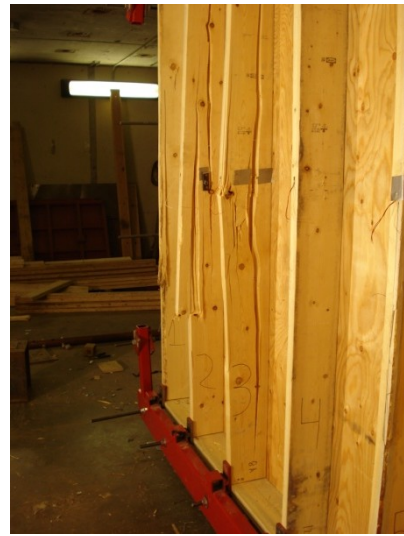
(c) Localized damage stud 1 to 3-Lower half
