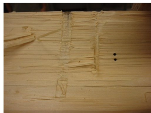
(c) Crushing of wood
