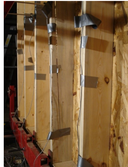
(c) Localize damage stud 4-Lower half
