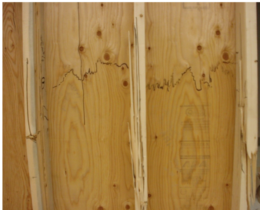
(b) Sheathing failure
