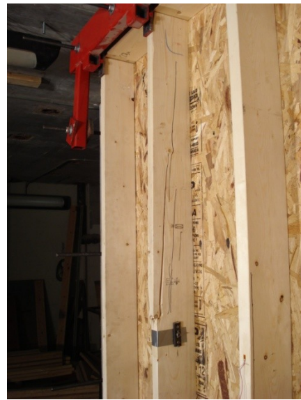
(c) Close-up of stud damage
