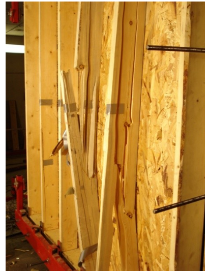
(c) Close-up of stud damage
