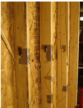
(c) Local damage
