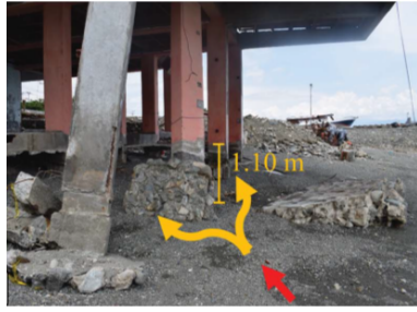
(a) Scour around columns in Watusampu
