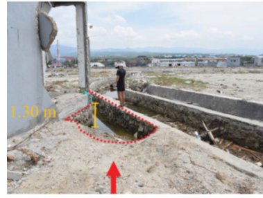
(b) Scour at southern corner of Shops
