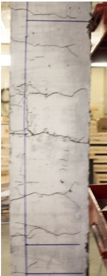
d) Mid-span cracking at Blast 2
