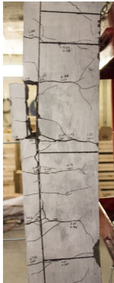
e) Mid-span spalling at Blast 2A
