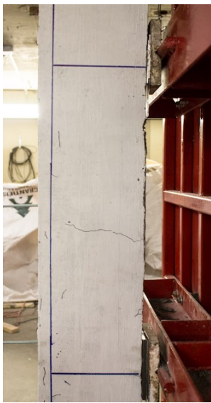
c) Mid-span hairline cracks at Blast 1
