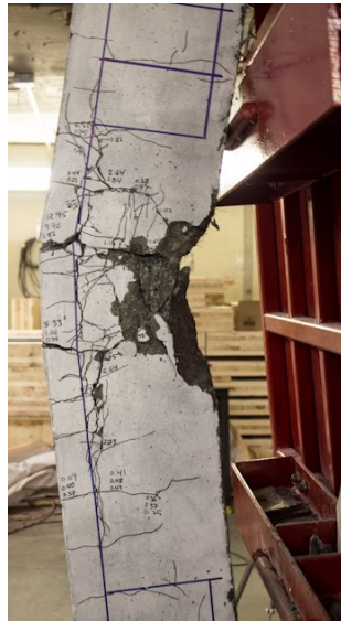
g) Mid-span crushing at Blast 5
