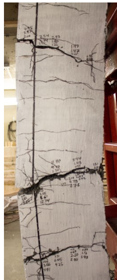
g) Mid-span splitting at Blast 3A
