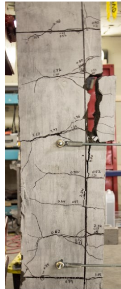
f) Mid-span spalling at Blast 2A
