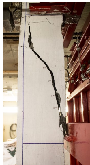
e) Shear-crack (top) at Blast 2
