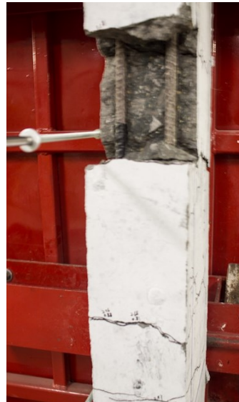
d) Mid-span spall at Blast 2A, HSC-F0-#4-S
