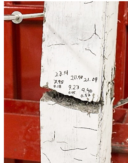
h) Mid-span fibre pulled out at Blast 5, HSC-F1(ZP)-20M-0
