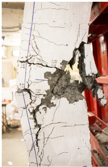
g) Mid-span crushing at Blast 5
