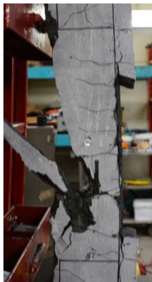
f) Mid-span cracking at Blast 4
