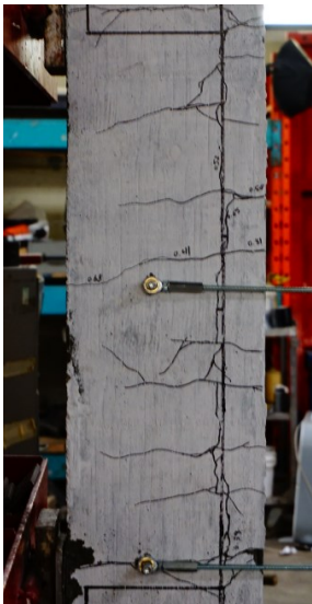
e) Mid-span cracking at Blast 3a
