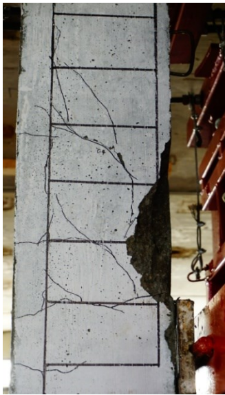
e) Top-span cracking at Blast 3b
