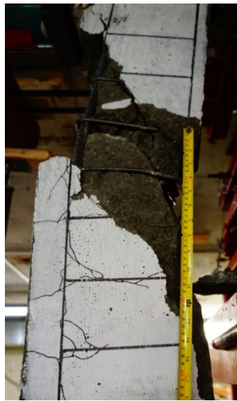
f) Top-span cracking at Blast 4
