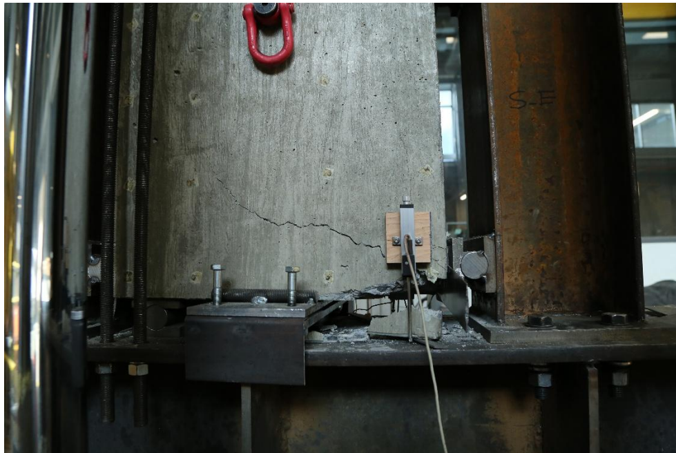
Figure 4-30: Crack induced by shim plates in the bottom right support.
