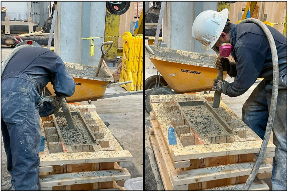
Figure 4-23: Beam-end internal and external vibration.
