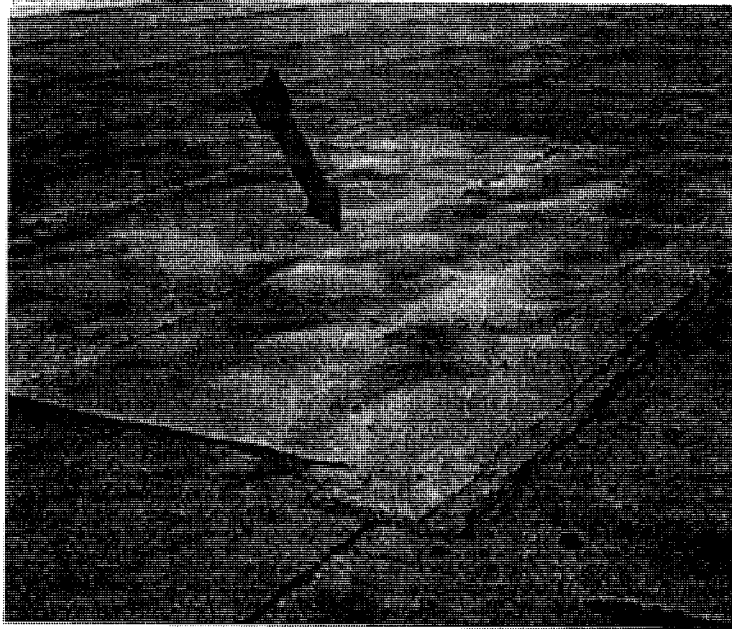
Figure 1.7 Development of blisters on roof assemblies ( www.waynesroofing.com )
