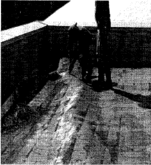
(a) Membrane lift up and sag
