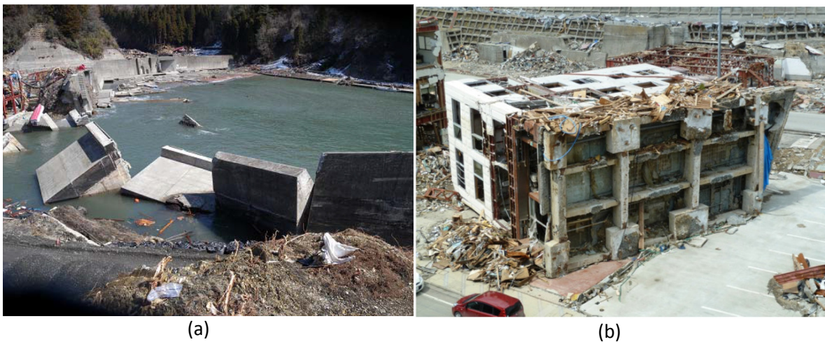
Figure 1.2: Destruction of nearshore structures during the 2011 Tohoku tsunami: (a) collapsed seawall at Ryoishi in Kamaishi (Takahasi et al., 2011) and (b) overturned concrete structure in Oganawa City, Myagi Prefecture (Courtesy of Dr. Ioan Nistor).
