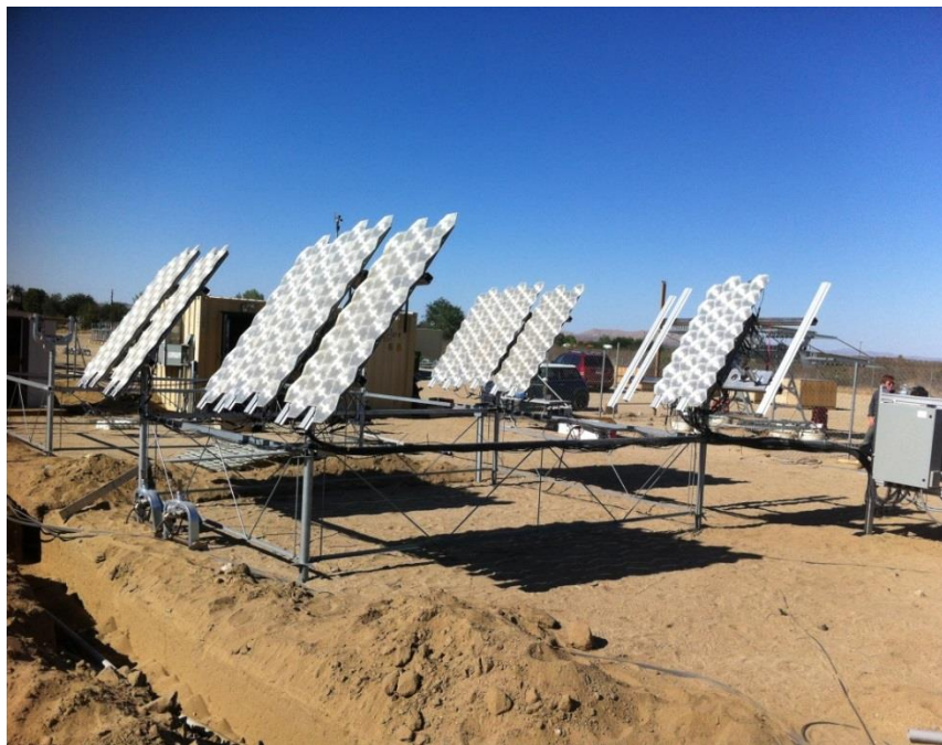
Figure 2-11: Implementation of Morgan Solar's Gen III LSO optic panels on a box-frame tracker.
