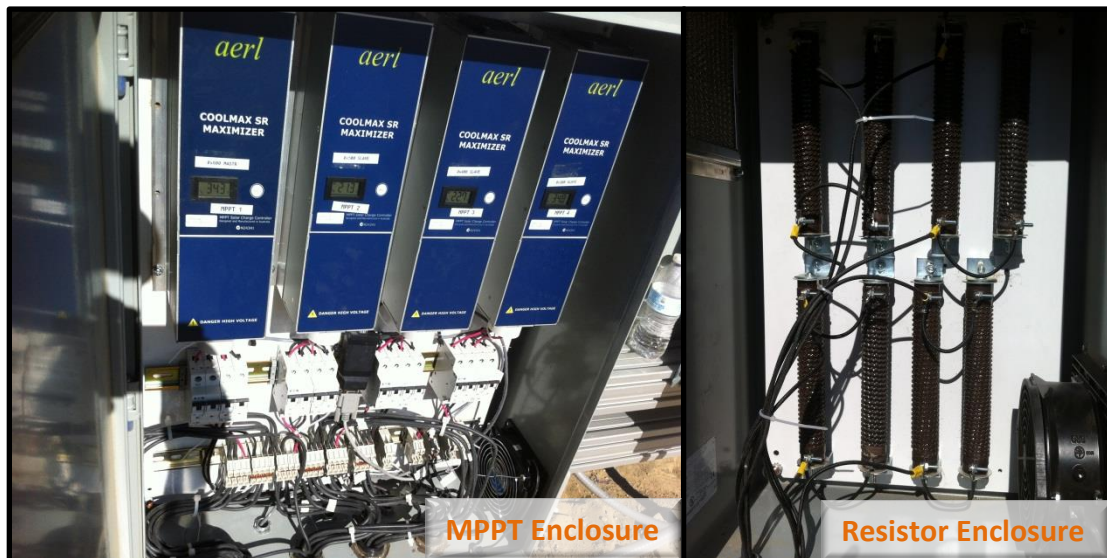
Figure 4-22: On left is the MPPT enclosure containing the AERL SRMVW MPPTs and the associated circuit breakers and terminal blocks. Shown on the left is the resistor containing the power resistors and cooling fan.
