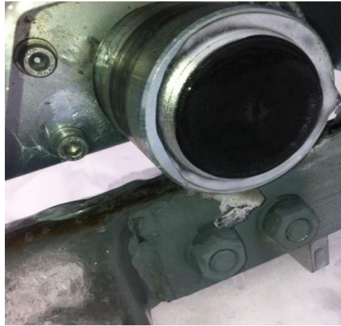
Figure 4-8: Ice build-up on tracker rail resulting in tracker failure. The tracker was unable to rotate in azimuth.
