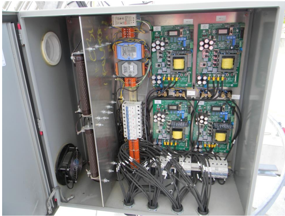
Figure 4-17: Fully assembled DC load. The four MPPT's, circuit breakers, terminal blocks, and the SuperLogics measurement devices are seen on the right side of the enclosure. The cooling fan and power resistors can be seen on the left.
