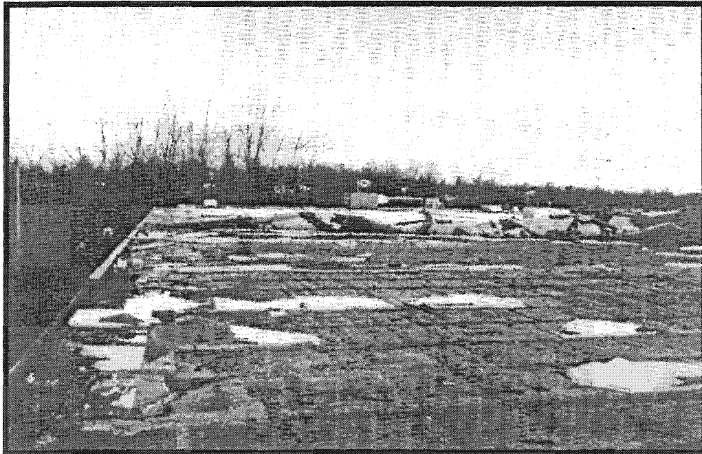
Figure 1.1 Roof failure during high wind event
