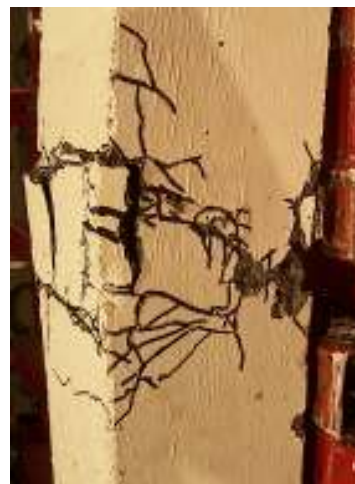
(c) Mid-Span Result of Blast 3
