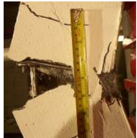
(c)Mid-Span Result of Blast 4(2)
