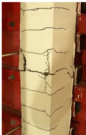
(a) Mid-Span Result of Blast 3
