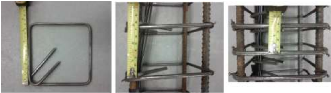
Figure 3.5 Typical (left) hoops and spacing of ties in (left) non-seismic and (right) seismic columns
