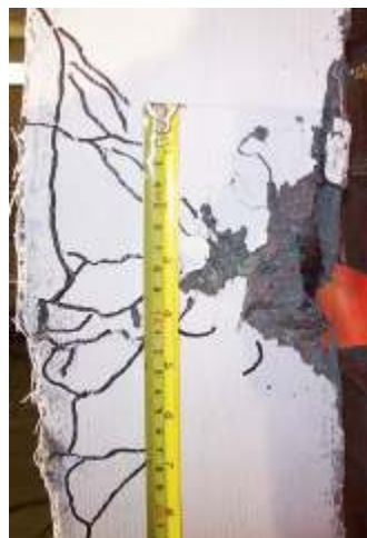
(a)Mid-Span Result of Blast 3
