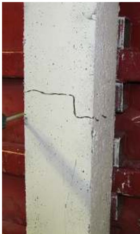
(a) Mid-Span Result of Blast 2
