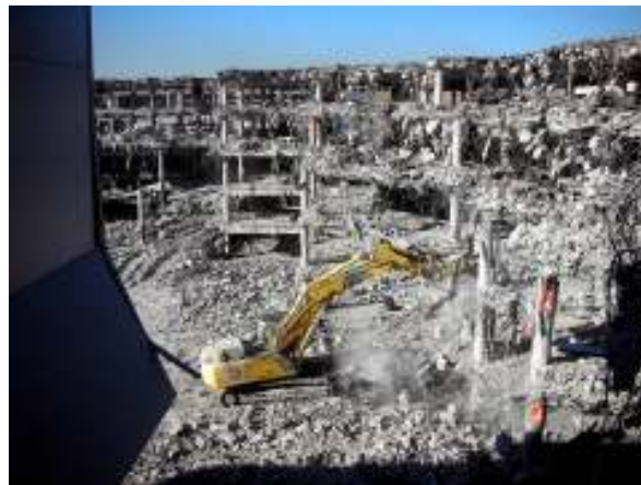
Figure 1.3 Effects of the 500kg explosive on the RC parking structure of Terminal 4
