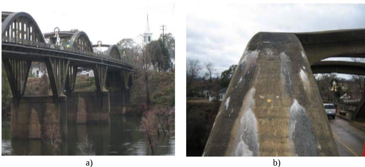
Figure 3.1: Bibb Graves Bridge. a) north face. b) cracking on of archway supporting the fifth span. Wetumpka, Alabama. Adapted from [4].
