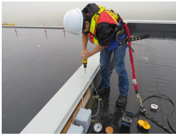
Figure 3.18: Drilling the hole for the pressure tap on the top face (Courtesy of Laith Hajsaid, University of Ottawa)
