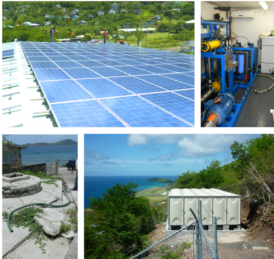
Figure 3. Images of the solar-powered desalination plant project in Paget Farm. Top left: Solar panels located on the hangar of the J.F. Mitchell Airport (image courtesy of M. Bento). Top right: Reverse osmosis desalination system. Bottom left: One of three desalinated water outlet. Bottom right: The 20,000 gallon water holding tank.
