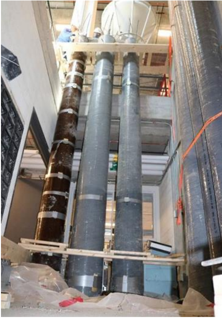
(a) Using a concrete pouring bucket to pour the concrete into the towers
