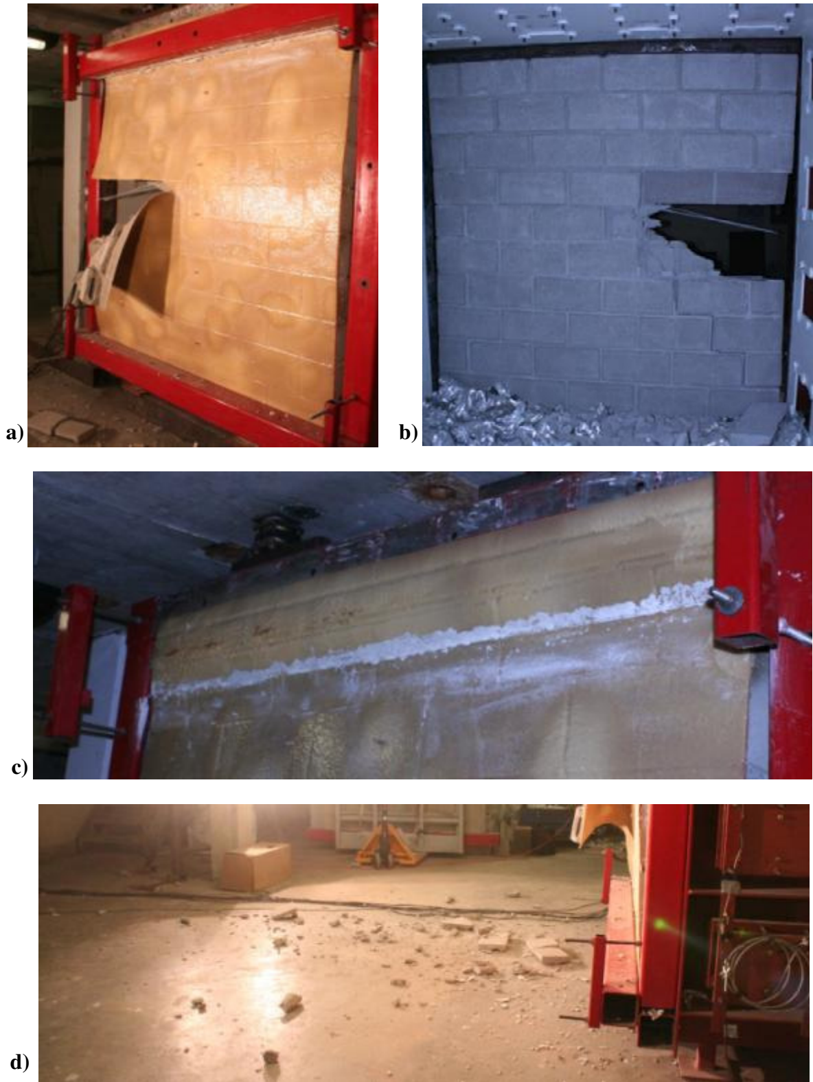
Figure 3.31: Retrofitted Infill Wall URM-2 after Shot 10: a) Extended Tear in Polyurea; b) Compression Face of the Wall; c) Extended Debonding at Supports; d) Scattered Debris after Global Failure of Specimen
