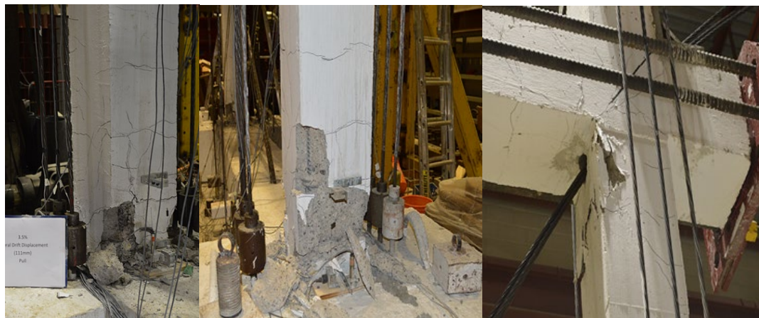
Figure III-7 Increased cover concrete crushing and crack pattern at 3.5 % drift during
