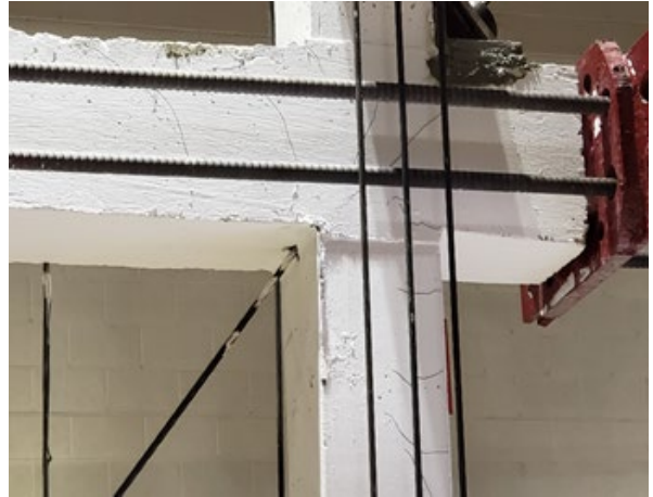
(b) East beam-column joint
