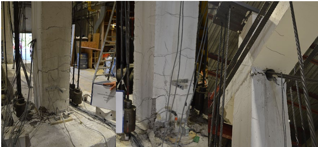
Figure III-6 Increased cover concrete crushing and crack pattern at 3.0 % drift during Test 2
