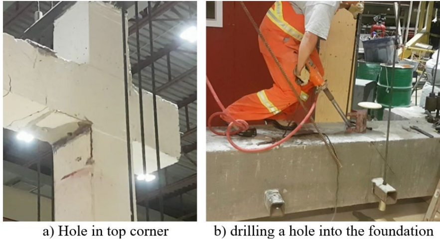
Figure 4-17 Preparation of the new foundation to facilitate the placement of diagonal strands
