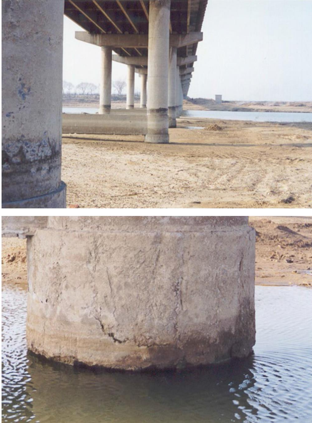
Figure 1.1. Concrete piers of a highway bridge subject to frost damage (reproduced from Li 2016)
