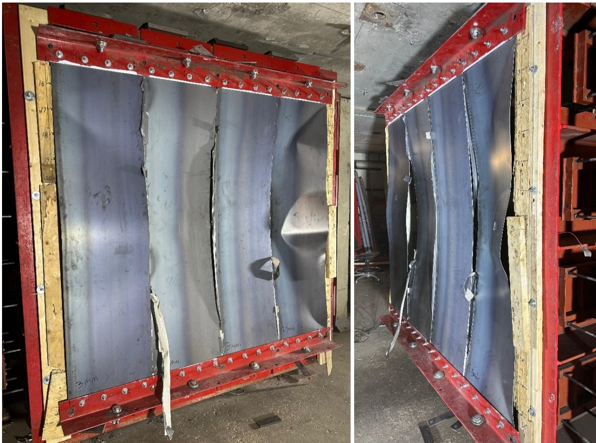
Figure 89: Buckling of steel sheets after shot #2
