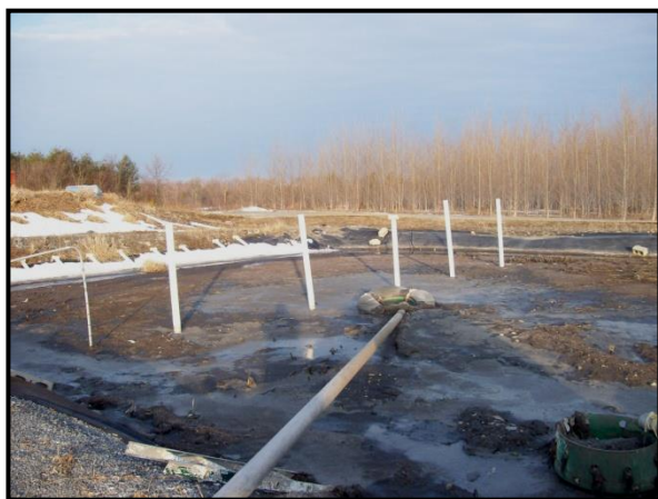
Sand Filter operating as a freezing bed (12)
