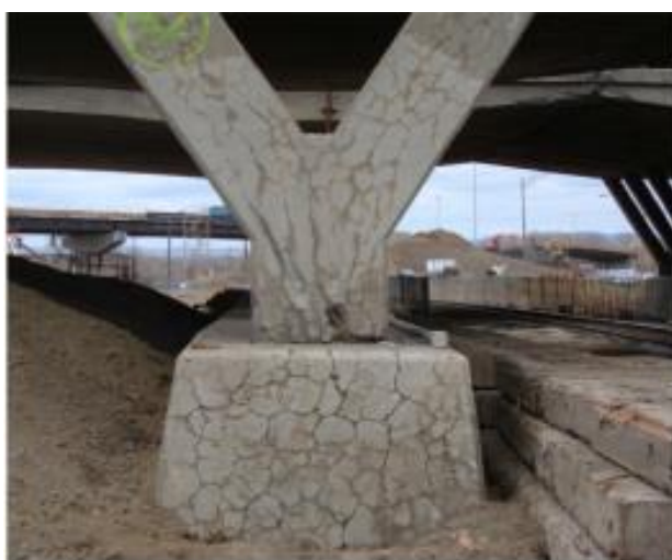
Figure 2.5: Severely affected concrete structure [32].
