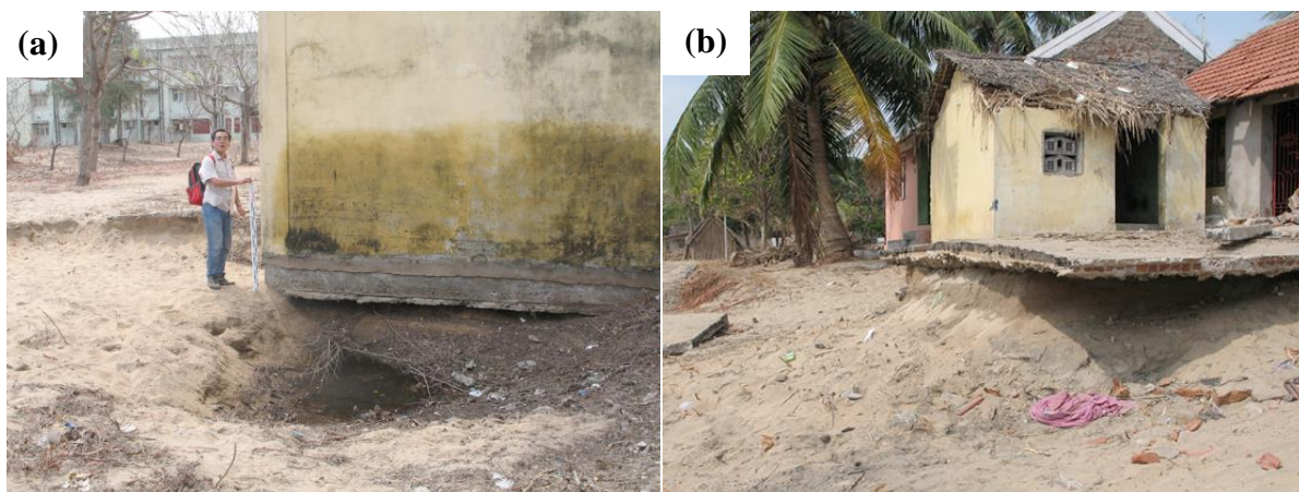
Figure 2.6: Local scour during the 2004 Indian Tsunami. (a) 1.4m Deep.(b) 1.5m Deep (Yeh and Li, 2008)
