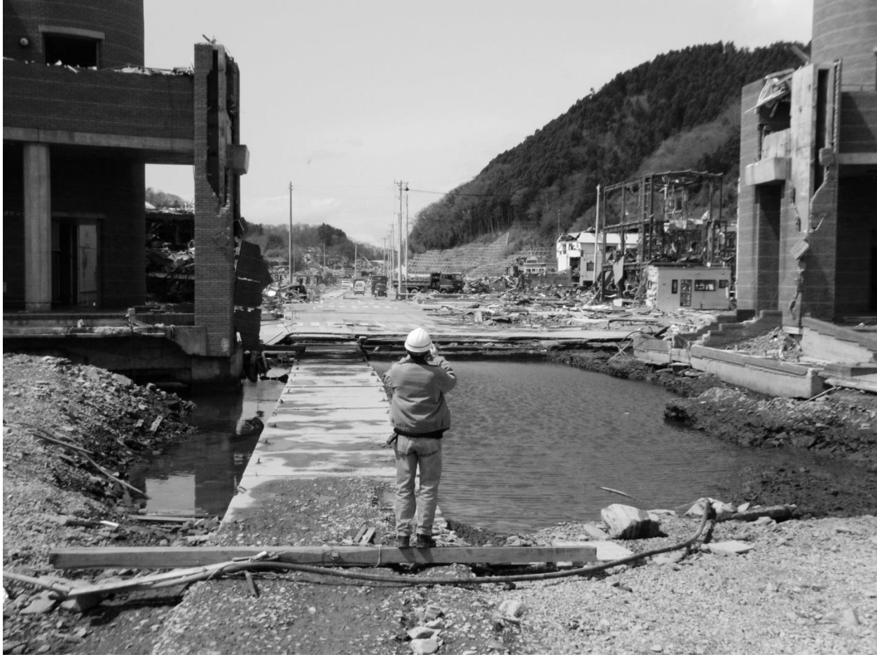
Figure 4.1: Deep scour hole between two hospital buildings in Oganawa caused by the 2011 Great Japan Tsunami
