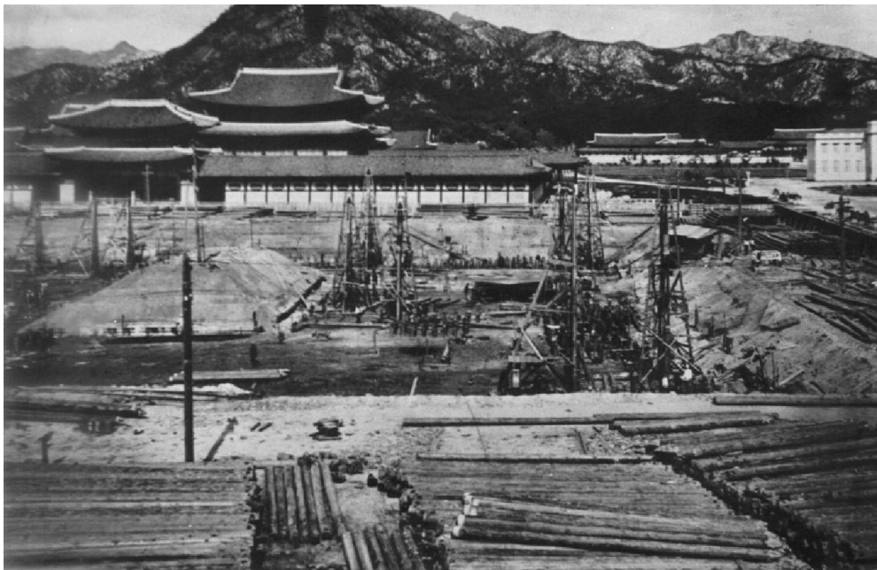
Figure 6. The construction site of JGGB in unknown year. Source: National Archives of Korea ( http://theme.archives.go.kr/next/koreaOfRecord/joseonChong.do )
