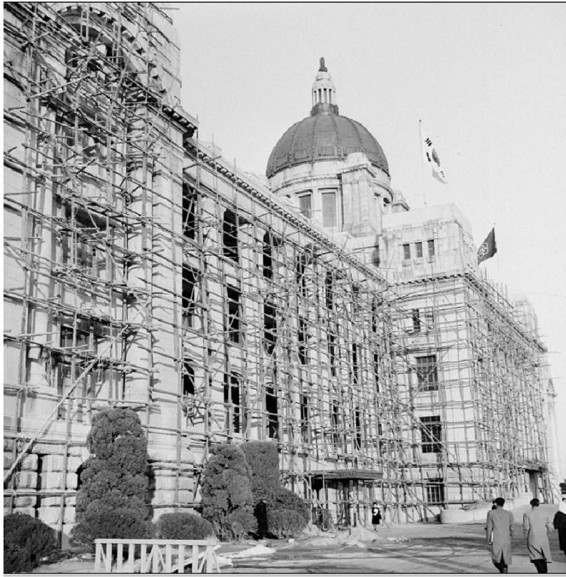
Figure 10. Repairing the inside of Capital Hall in 1962. Source: National Archives of Korea ( http://theme.archives.go.kr/next/koreaOfRecord/joseonChong.do )
