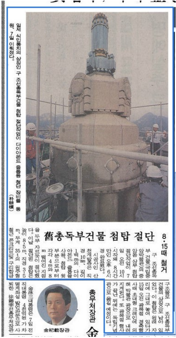
Figure 15. The cut spire of JGGB. Source: Gu Chong-Dok-Bu-Geon-Mul Cheom-Top Jeol-Dan [Cut the spire of former Japanese General Government building]. (1995).
