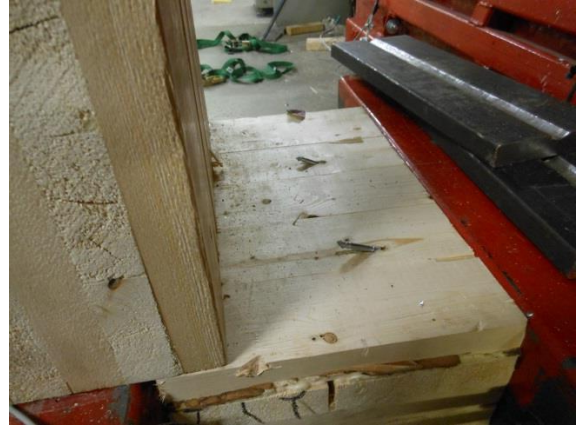
B) Failure of Bottom Connection Detailing
