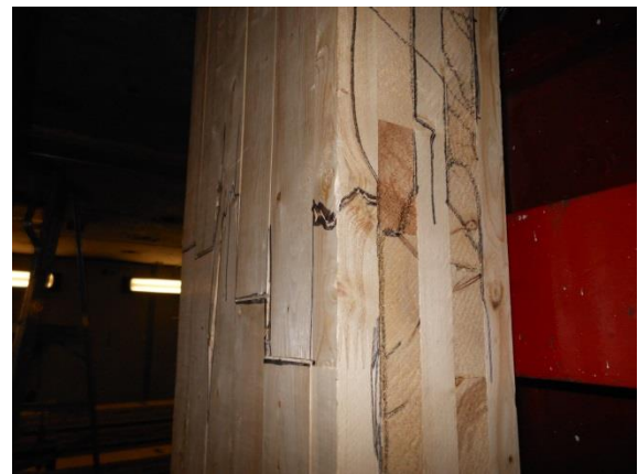
B) Right Side Flexural Failure
