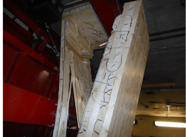
B) Top Tension Perpendicular to Grain Failure
