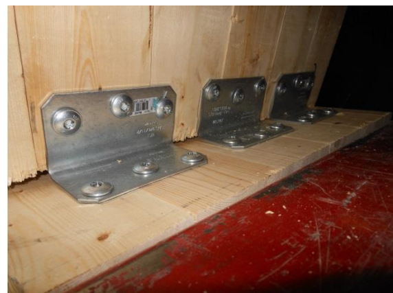
B) Close-Up of Bottom Steel Angles
