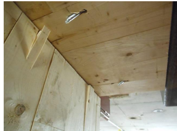
B) Failure of Top Connection Detailing
